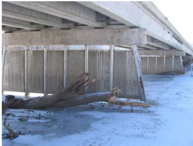
Figure 7.21: Bridge 23015 - upstream pier profiles and debris
