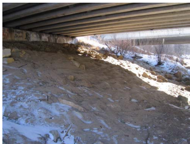
Figure 7.7: Bridge 6868/6869 - sand covered riprap on east abutment
