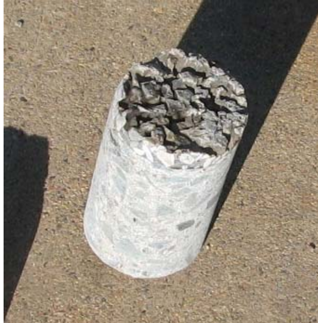
Figure 4.7. Photograph of core sample taken in September 2008. Location was at the edge of installation; outside of travel lane
