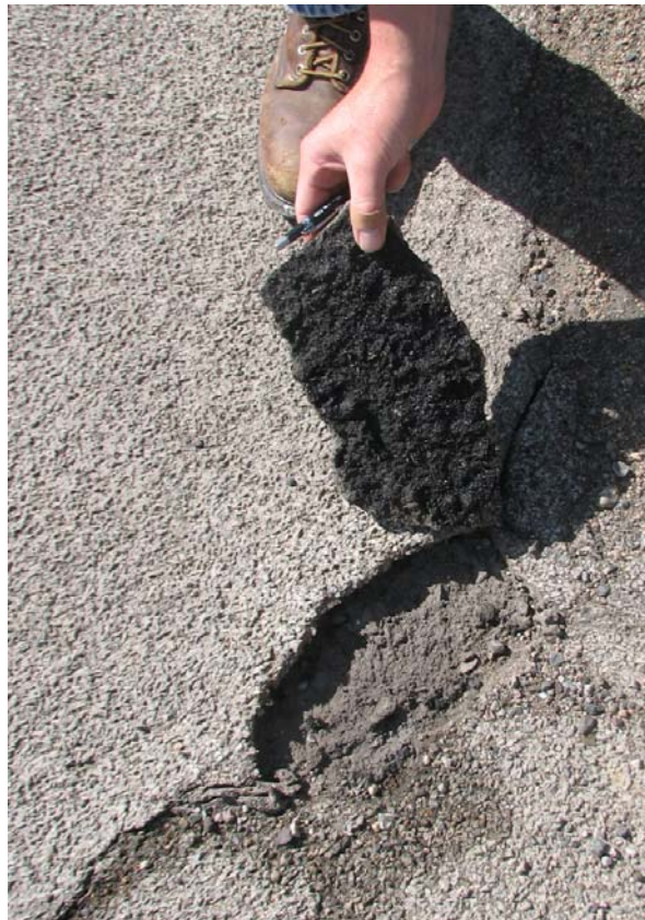
Figure 4.6. De-bonding over an asphalt repair patch.
