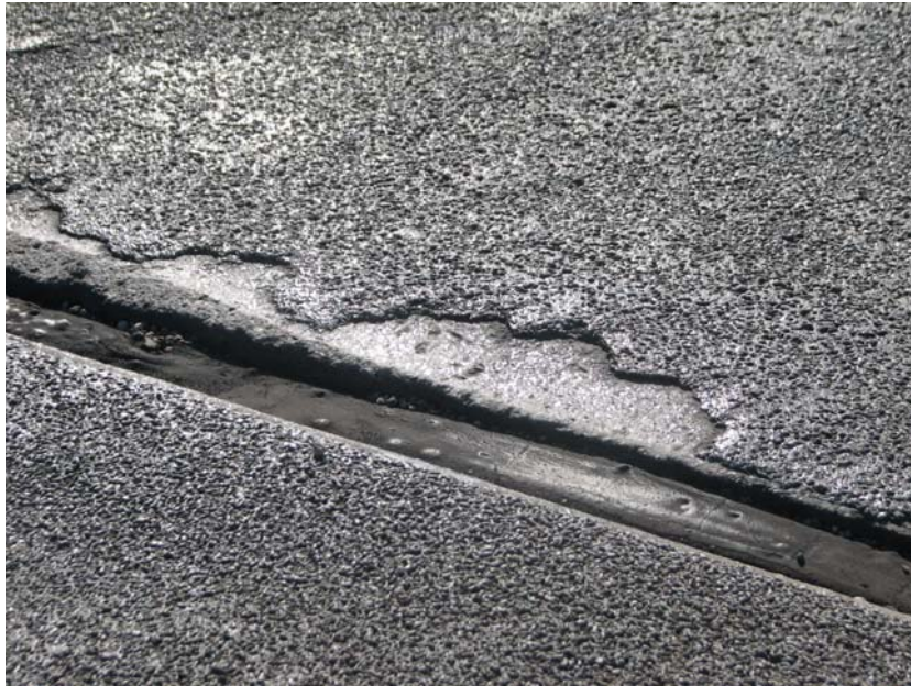
Figure 4.5. De-bonding at an expansion joint.
