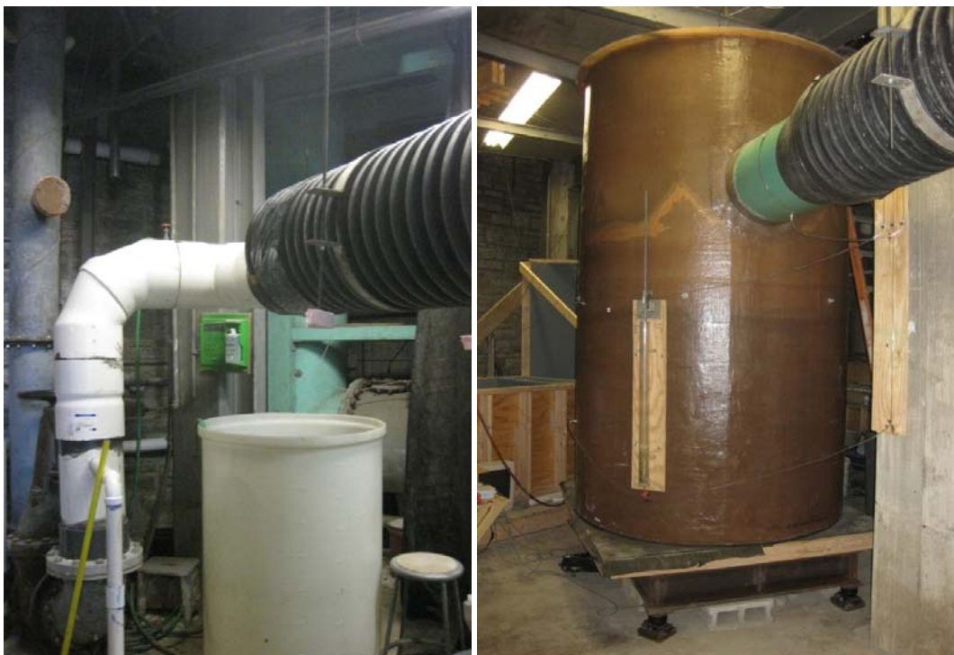
Figure A-11: Stormceptor water feed piping
