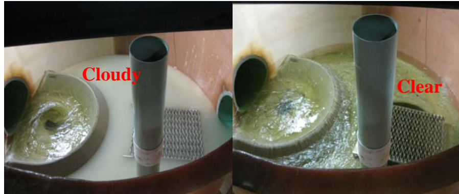
Figure 3-4: Cloudy and clear water on top of insert in Stormceptor
