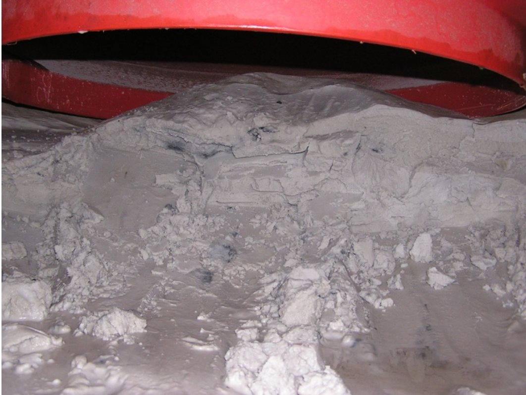
Figure 3-7: Sediment cone near Downstream Defender benching skirt
