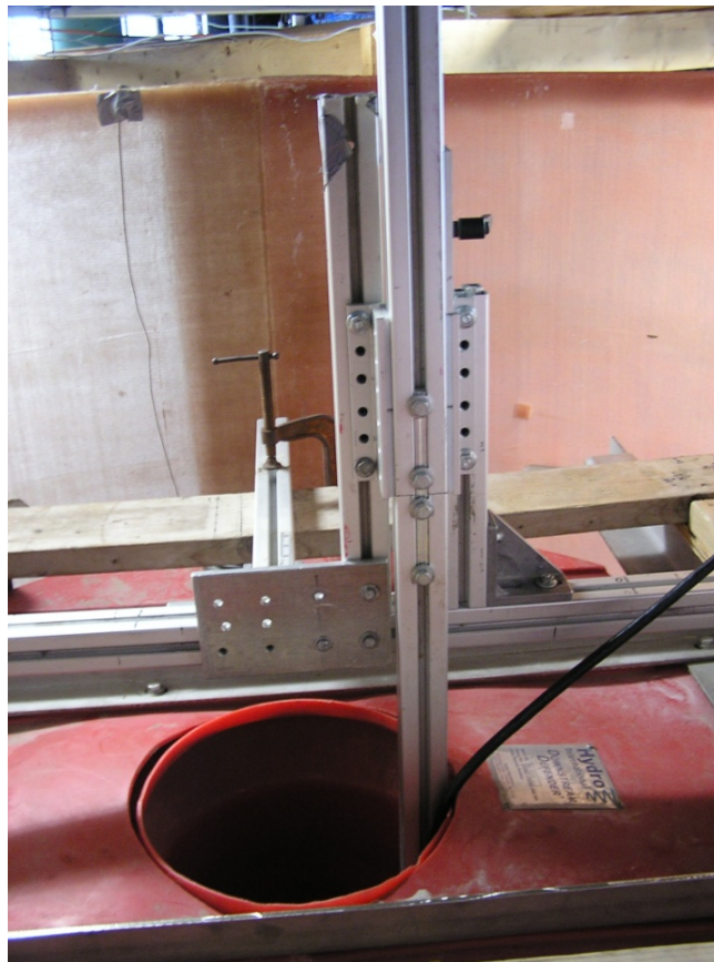
Figure 5-5: The ADV bracket installed on top of the Downstream Defender holding the ADV in the sump
