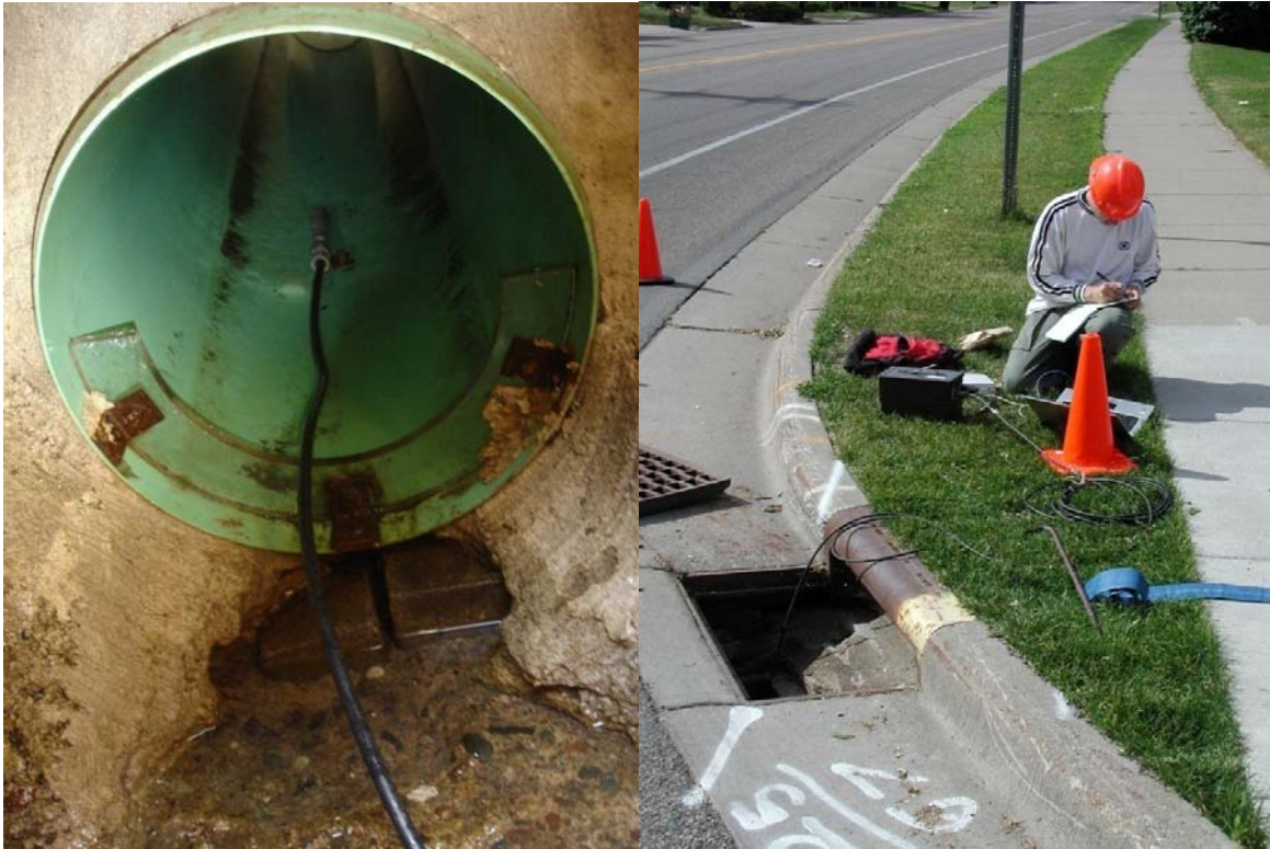
Figure A-4: Flow rate measurement using a weir, pressure transducer and data acquisition computer
