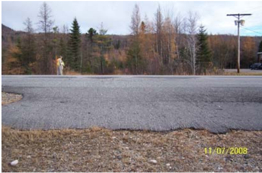
US Route 3 Approach Apron Surface Wear, Minor Loss of Edge
