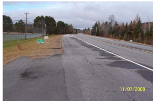
US Route 3 Approach Apron Surface Wear, Limited Loss of Edge
