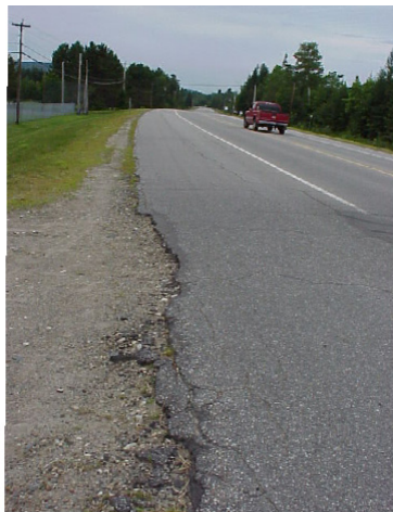
Fig. 1 -- Southbound shoulder edge is broken from stud damage during snowmobile acceleration to cross highway.
