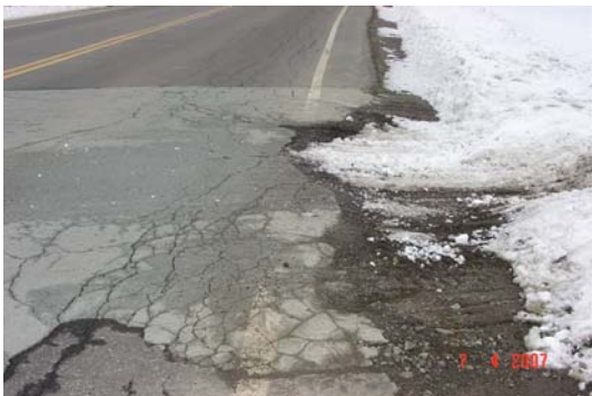
NH Route 26 Shoulder Erosion and Edge Chipping
