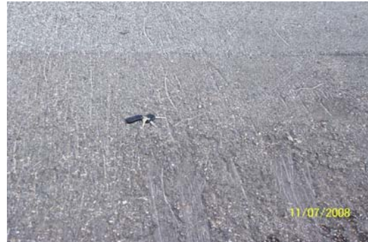
US Route 3 Approach Apron Surface Wear, No Loss of Edge
