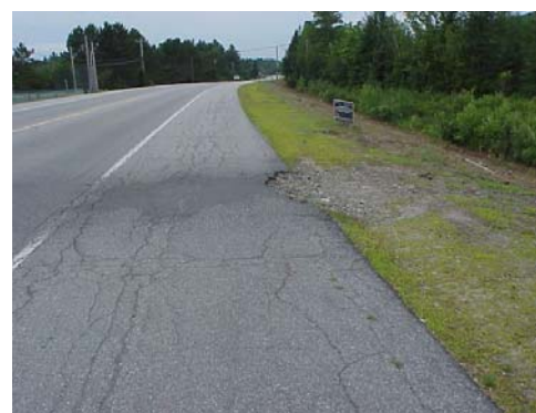
Fig. 2 – Northbound shoulder edge is broken and pavement surface is worn from snowmobile studs.
