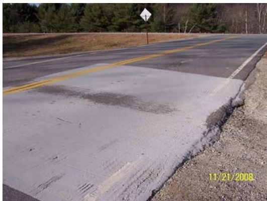
Halls Brook Road, Rumney Single-lane and Edge Wear (Note Steep Slope Grade and Erosion of Shoulder Materials)
