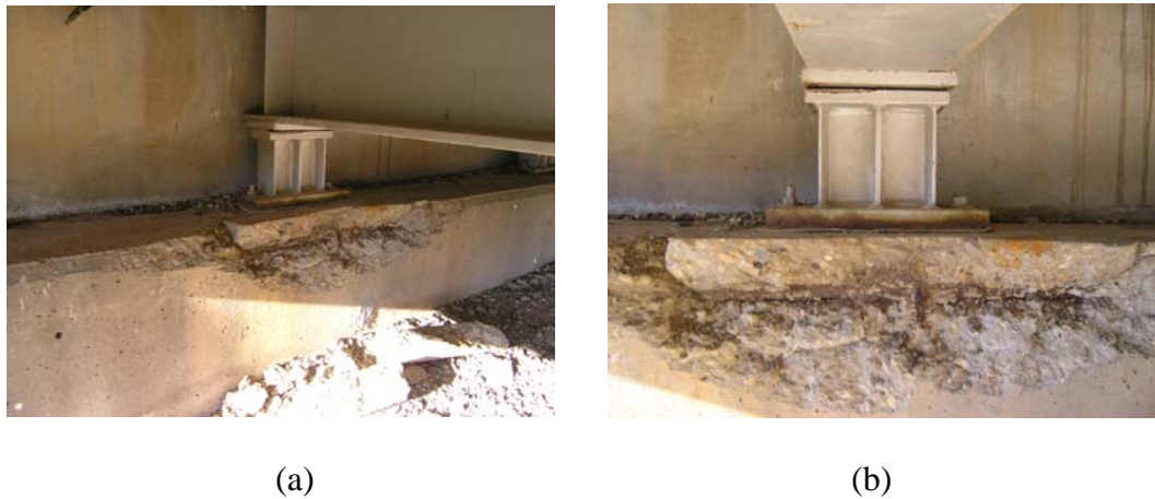
FIGURE A8 Spall with Exposed Rebar at Abutment: (a) Poor and (b) High Quality Picture.
