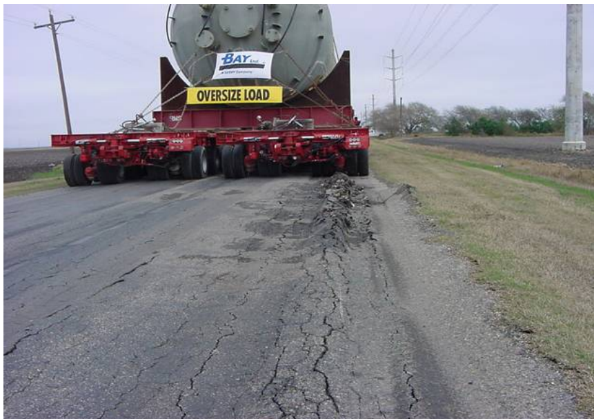
Figure 5. Severe Damage on FM 796.
