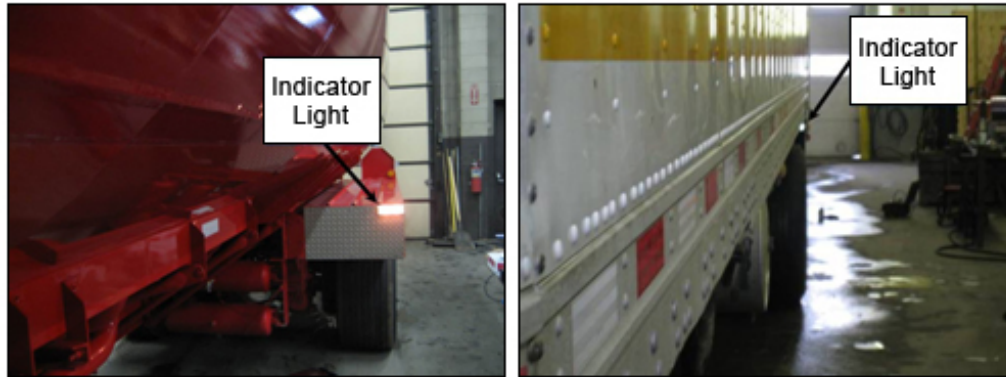
Figure 19. Grouped photo. CLI and GFS indicator light installation on the fender (left) and underside of the reefer pup (right).
