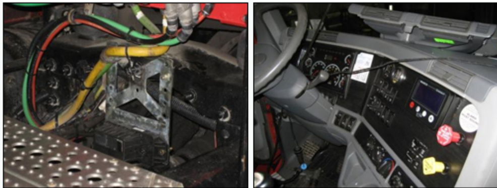
Figure 9. Grouped photo. ECU (left) and display unit (right) installations.
