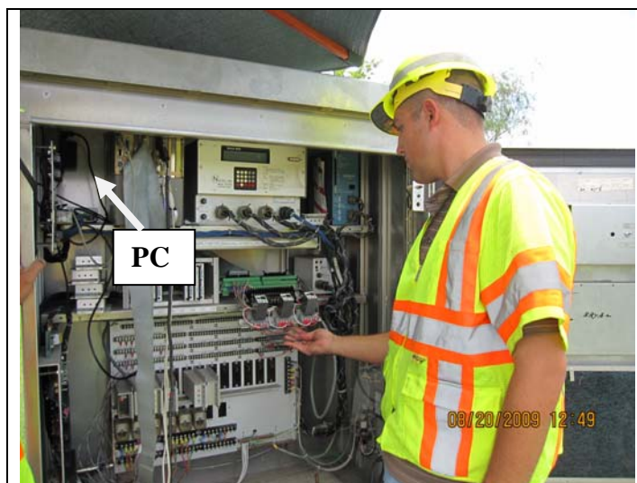
Figure 6. Equipment Installed in Caldwell Controller Cabinet.
