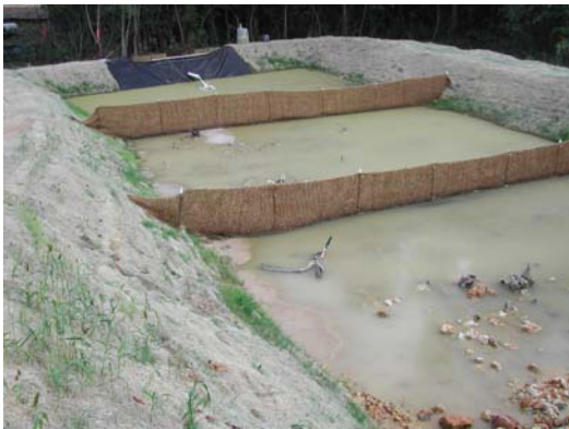
Figure 3. Skimmer Basin 2 (SkB2) with coir baffles
