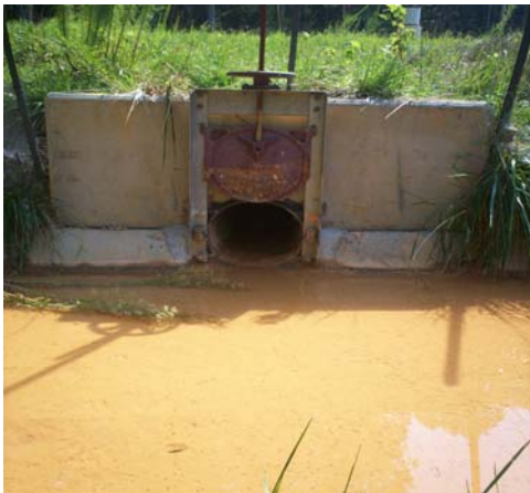
Figure 17. Level spreader at outflow of skimmer. Not maintained and full of sediment backing up into discharge pipe.
