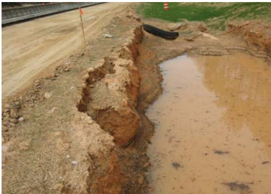
Figure 13. Standard Trap with standing pool 2 (STSP2) with weakened vertical walls.
