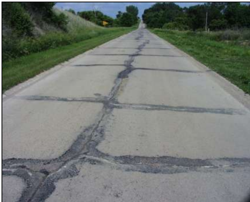
Figure 52 - Old U.S. 20 Woodbury County 1921 - no jointing
