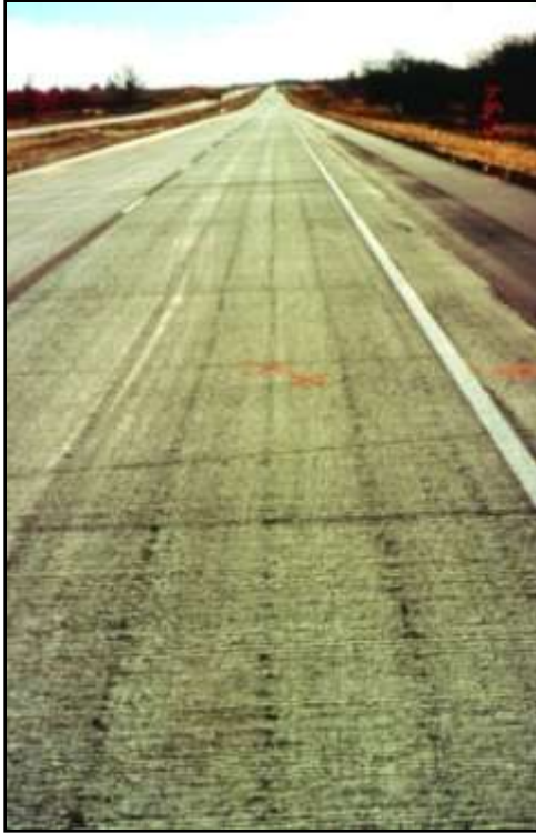
Figure 38 - Vibrator trails in pavement - Dallas County
