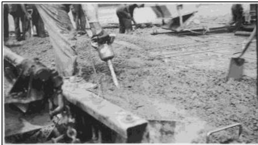
Figure 36 - Vibration near expansion joint - Bremer County 1936
