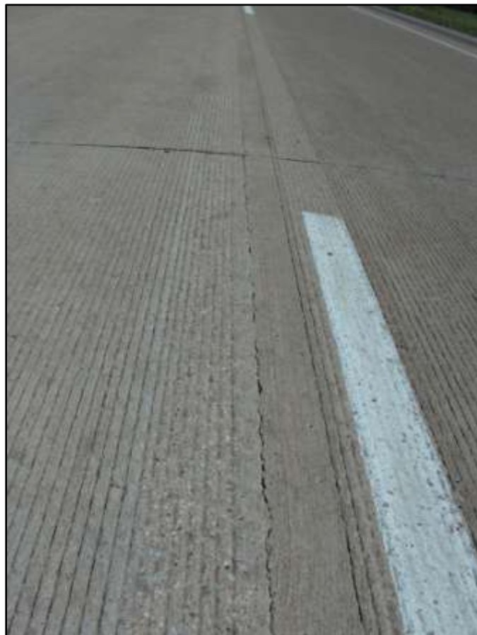
Figure 62 - Hairline crack on knifed joint
