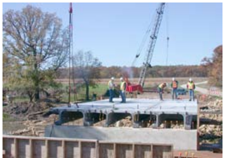
Figure 30 - Pi-girder span of the bridge under construction; three individual pi girders were placed before being connected to each other.
