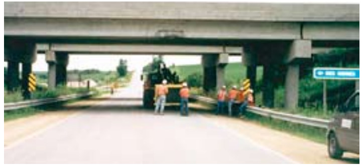
Figure 17 - View of damaged exterior girder in the center span of the Beebeetown bridge, westbound on I-680 in western Iowa; damage was restricted to the exterior and first interior prestressed girders.
