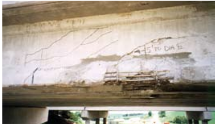
Figure 18 - Close-up view of damaged exterior and interior girders; the damage included loss of section properties and severe cracking, as well as damage to prestressed strands.
