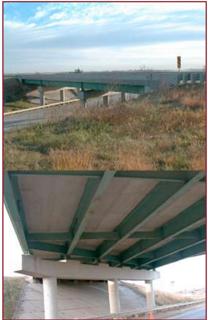
Figure 21 - A multiple steel-stringer bridge on I-35 in southern Iowa; several web gap locations and associated diaphragms were monitored during a diagnostic load test before and after an implemented retrofit.
