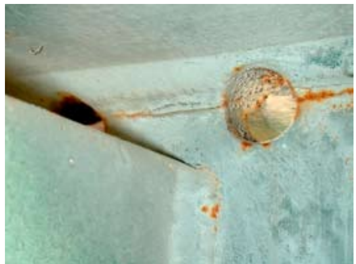
Figure 22 - A web gap on the I-35 bridge showing previously developed cracks; for the initial retrofit, holes were drilled at the ends of the crack. However, cracking continued to spread beyond the hole retrofit.
