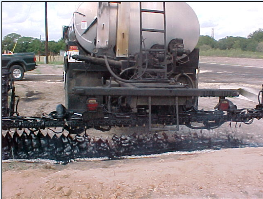
Figure 3 – Blowing Out Spray Bar
