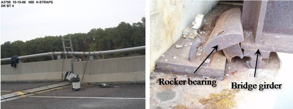
Figure 1. Photographs of a bridge that fell off its rocker bearings due to pier displacements
