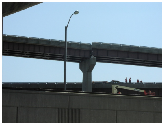
Figure 2. Bridge in New York that has fallen off its bearing and come to rest on the pier cap.
