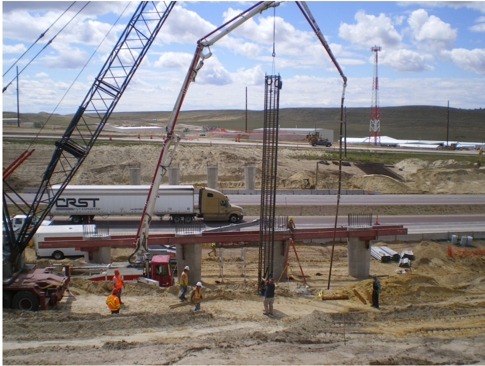
Figure 11. Concrete placement in the bottom of the shaft prior to placement of the reinforcing cage (Photo by S. Cooney)
