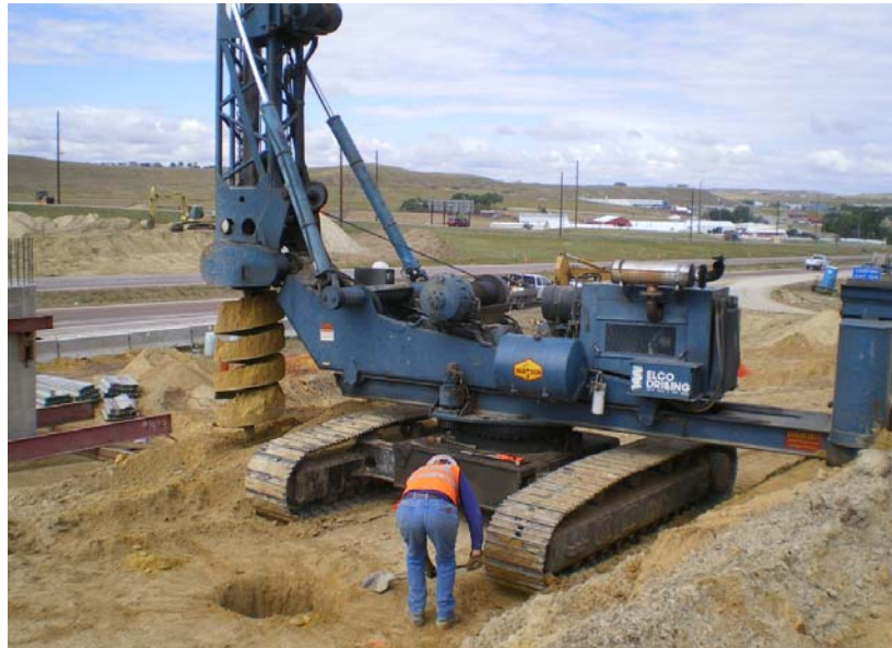
Figure 8. Drilling operation for installation of the test shaft (Photo by S. Cooney)
