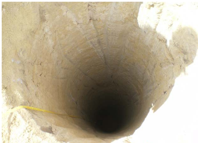
Figure 9. Photo of the drilled shaft borehole prior to concrete placement (Photo by S. Cooney)
