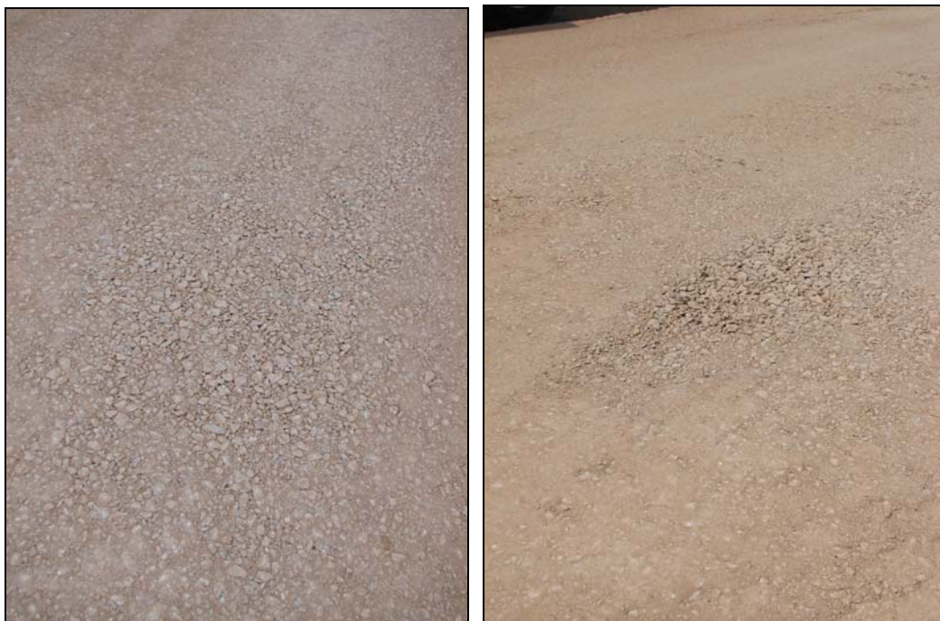
Figure 2.15. Segregation of Grade 4 Base after Placement.
