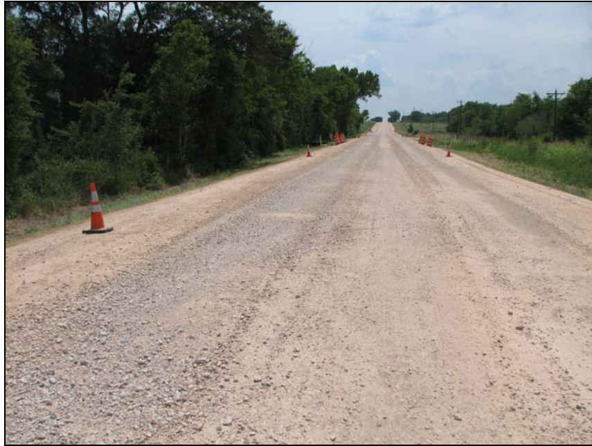
Figure 2.16. Raveling and Loss of Surface Finish of Grade 4 Base under Traffic.
