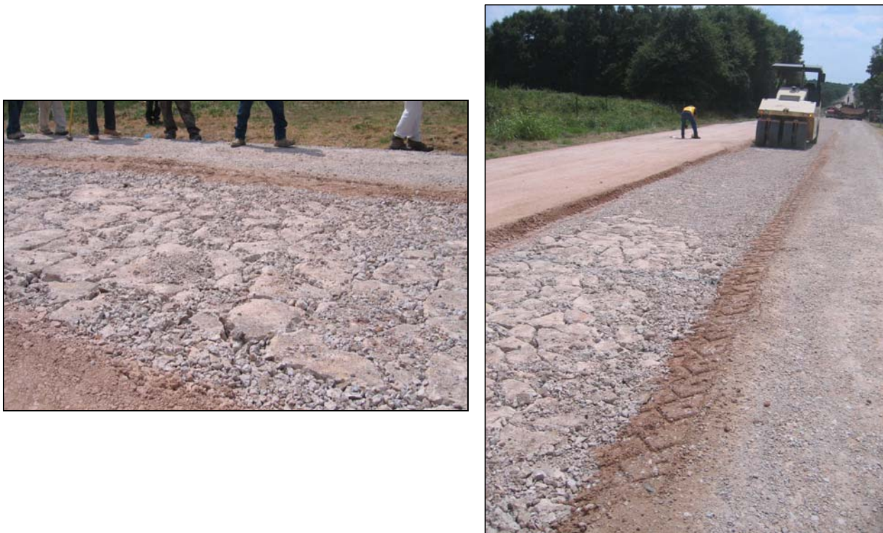
Figure 2.3. Poor Break Pattern at Unstable Location.
