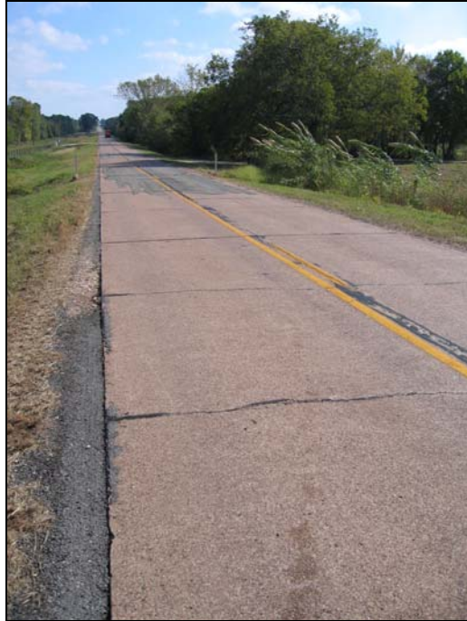
Figure C.1. Cracked Slabs on FM 912.
