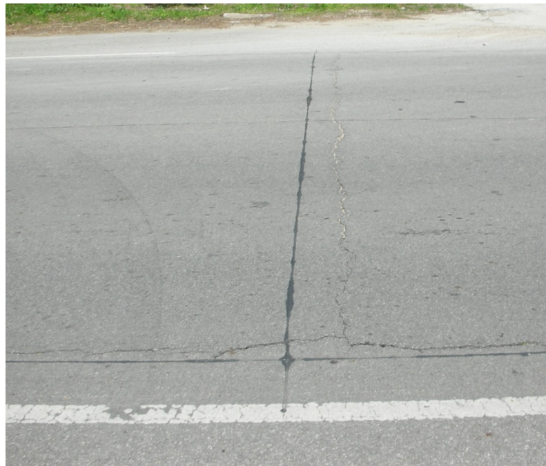
Figure 3-5. Cracking Parallel to Saw & Seal in May 2007.
