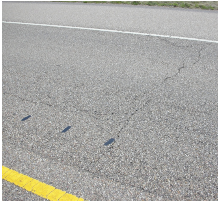
Figure 3-11. Typical Reflective Crack on Amarillo Test Pavement in 2007.
