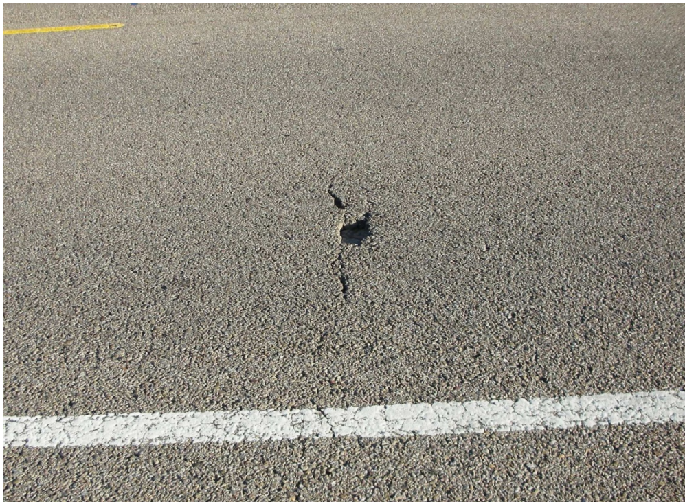
Figure 3-13. Pothole Observed in PaveTrac Section in 2006.
