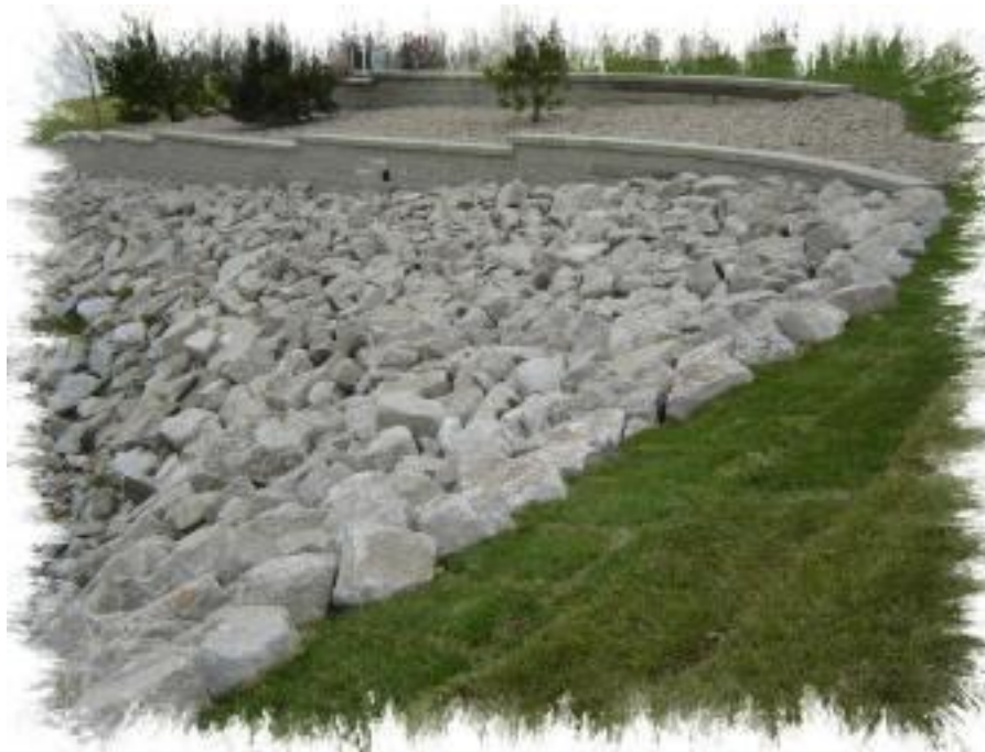
Figure 41: Photo of recycled concrete pavement used as “rip-rap” for erosion control (Photo courtesy of Blessing Construction, Kearney, NE).
