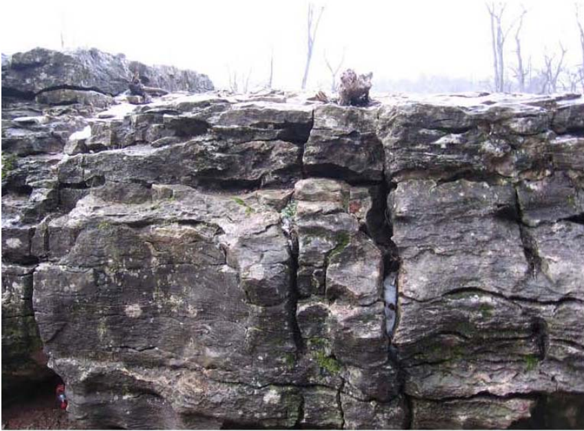
Figure 5: Outcropping Burlington-Keokuk limestone is typically dissected by solution-widened joints or faults. The ceiling of the access tunnel in underground limestone (~100 ft below the ground surface) is not characterized by prominent fractures (Figure 2).
