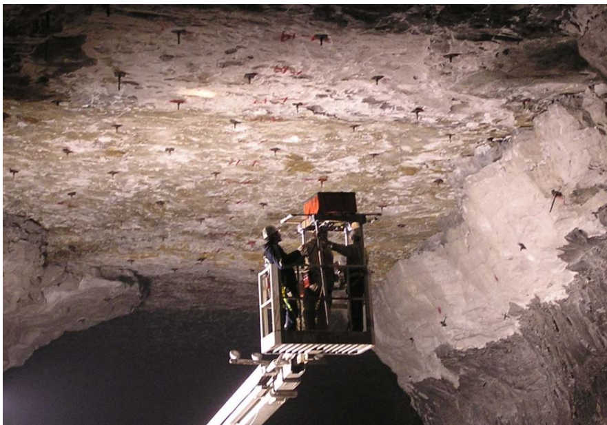
Figure 2: Photograph of ceiling of access tunnel several tens of feet to the west of the zone of failure. Newly installed rock bolts are observed. The crew is acquiring GPR data using a 200 MHz GSSI antenna in an effort to locate clay-filled solution-widened fractures.
