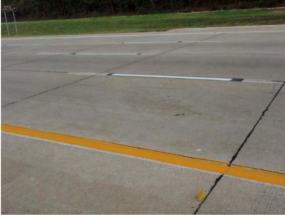
Figure 5 - MO 141 in St. Louis. Note all lines are newly applied and were painted in side grooved or milled slot in the concrete pavement.
