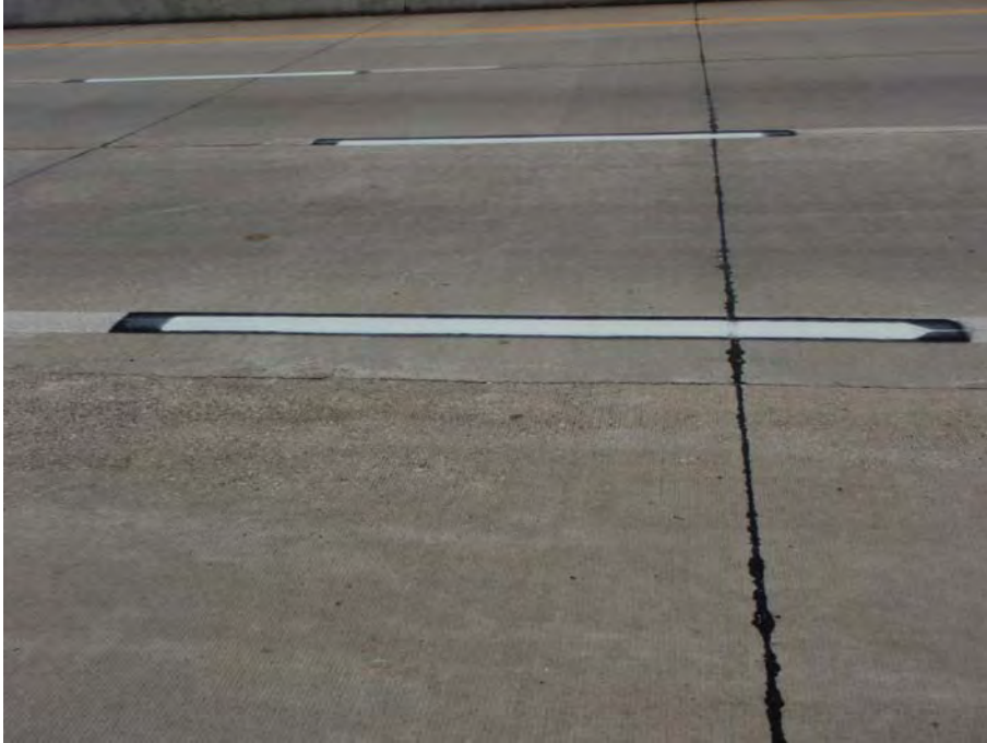
Figure 6 - Close up of dashed lane lines (skips): Note the black background paint applied within grooved area and white stripe well inside the borders meeting JSP 08-07 requirements.
