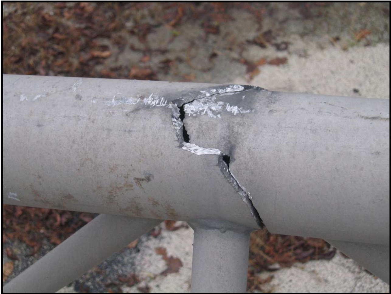
Figure 7: Additional Close-Up View of the Fractured Lower-Chord Connection
