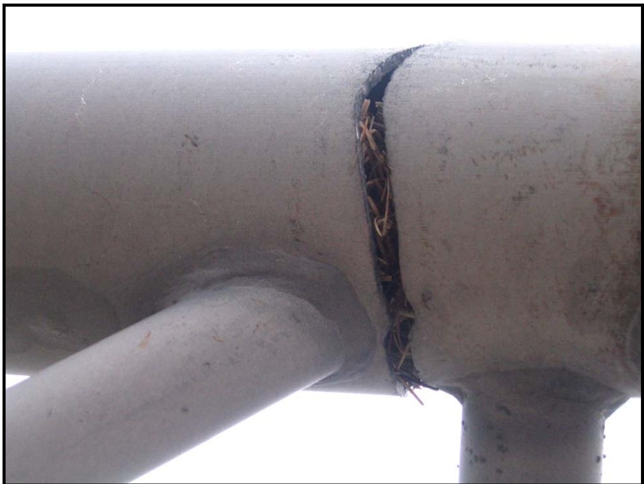
Figure 6: Close-Up View of Fractured Lower Chord Section
