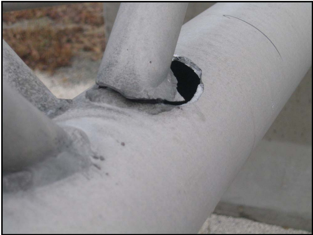
Figure 8: Close-Up View of the Failed Upper-Chord Connection
