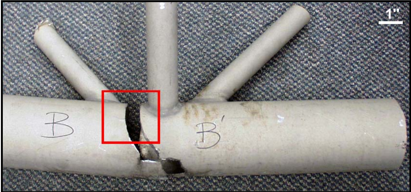
Figure 20: Sample B Taken From Failed Truss Lower Chord
