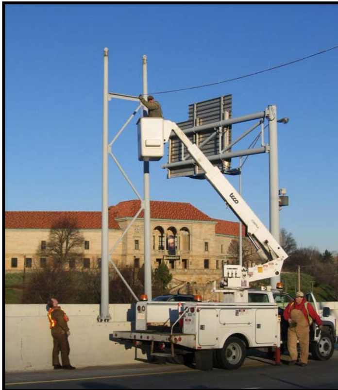
Figure 10: Instrumentation Cable Suspended Between Sign Towers
