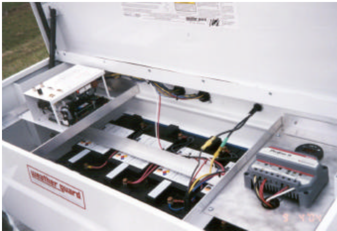
Figure 41: Inside view - battery box showing microcontroller at left, batteries at center, and power monitor at right
