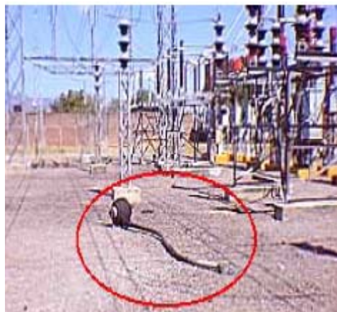
(e) Broken insulator
