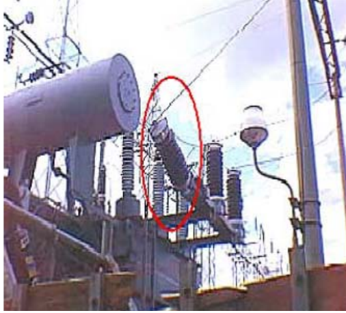
(a) Broken bushing of a transformer
