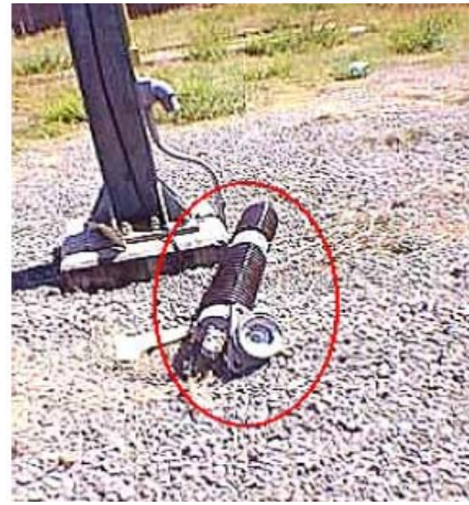
(b) Broken bushing of a lightning rod
