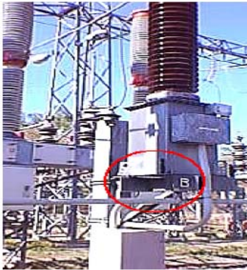
(c) Oil leakage from the bottom end of radiator
