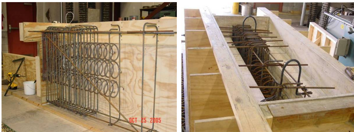
Figure 30 – (a) Open form with mild steel reinforcement; (b) Closed form with mild steel reinforcement and lifting hooks
