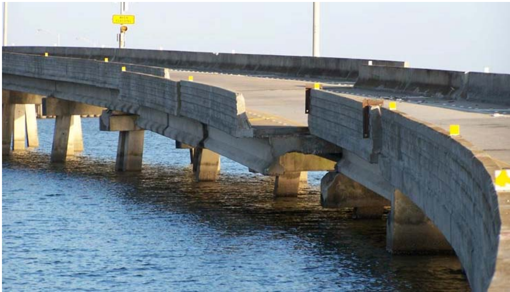
Figure 1- 8 I-10 Mobile Bay Bridge onramp spans displaced by Hurricane Katrina.
