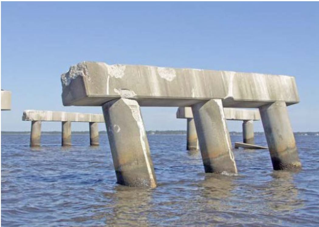
Figure 1- 6 I-10 - Escambia Bay Bridge pile bents damaged by Hurricane Ivan.
