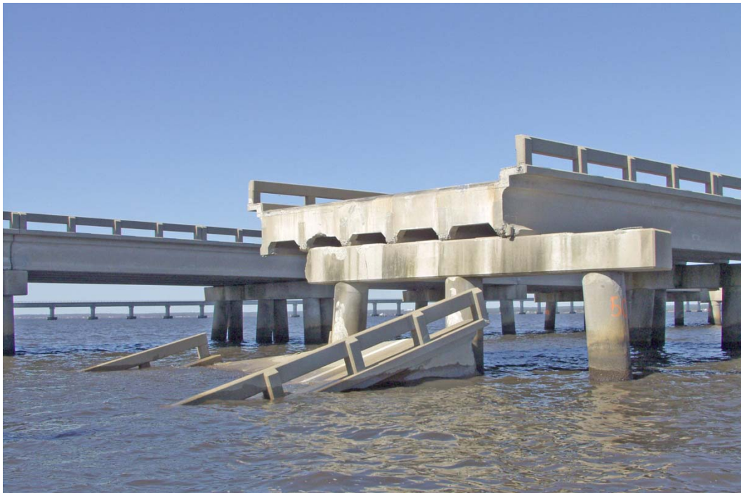
Figure 1- 4 I-10 - Escambia Bay Bridge spans removed by Hurricane Ivan.
