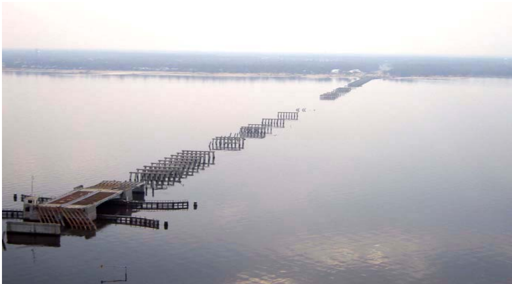
Figure 1- 14 US 90 - St. Louis Bay Bridge damaged by Hurricane Katrina.
