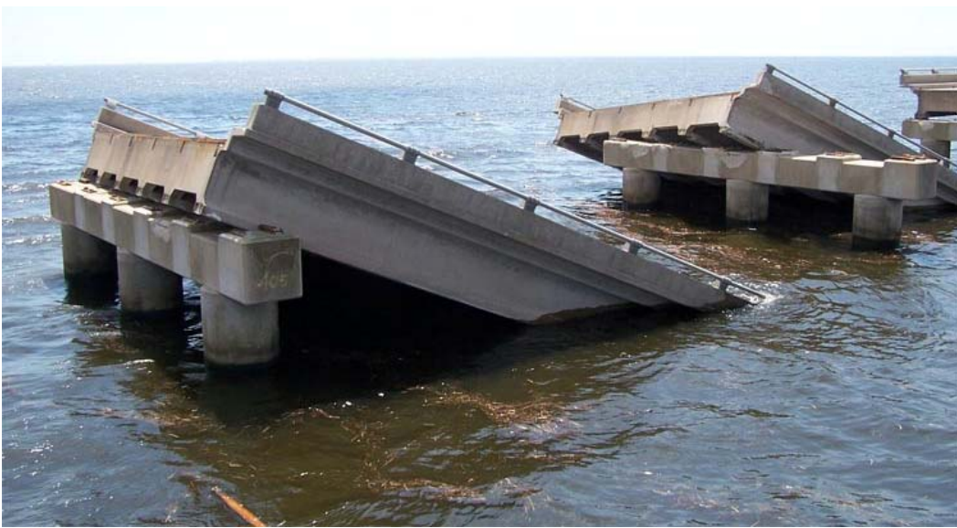
Figure 1- 11 I-10 Lake Pontchartrain Bridge support structures damaged by Hurricane Katrina.
