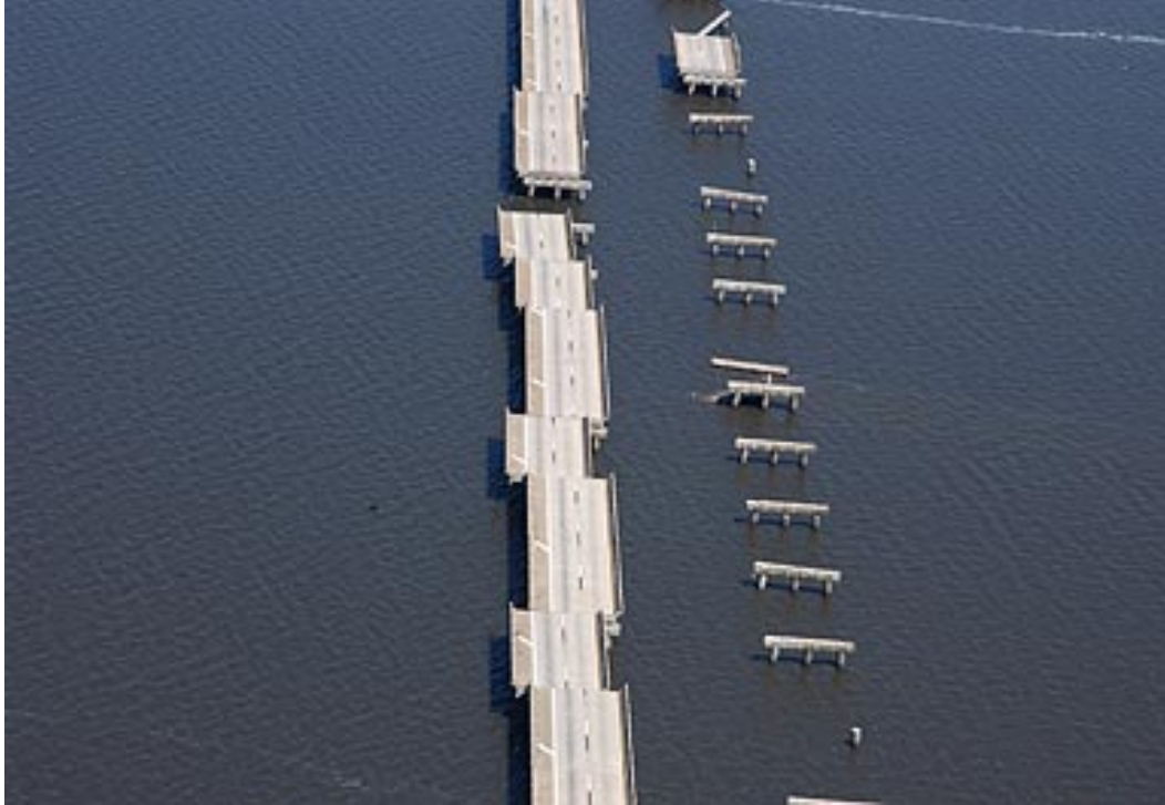
Figure 1- 3 I-10 - Escambia Bay Bridge damage from Hurricane Ivan.
