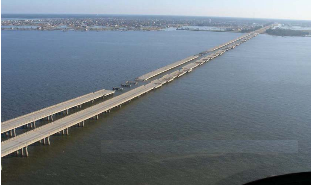
Figure 1- 9 I-10 - Lake Pontchartrain Bridge damage from Hurricane Katrina.
