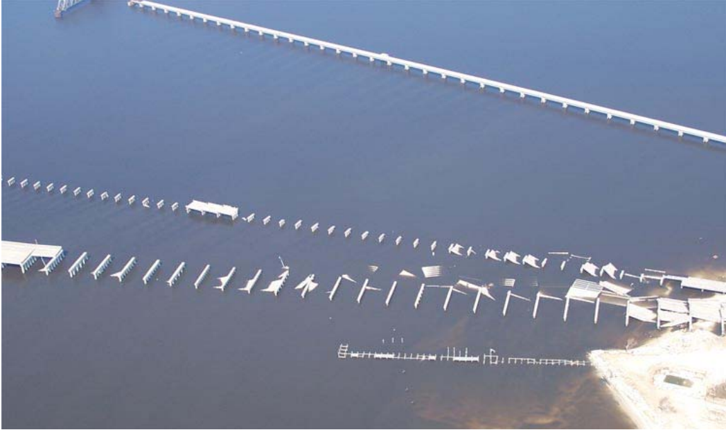
Figure 1- 13 US 90 - Biloxi Bay Bridge damaged by Hurricane Katrina.
