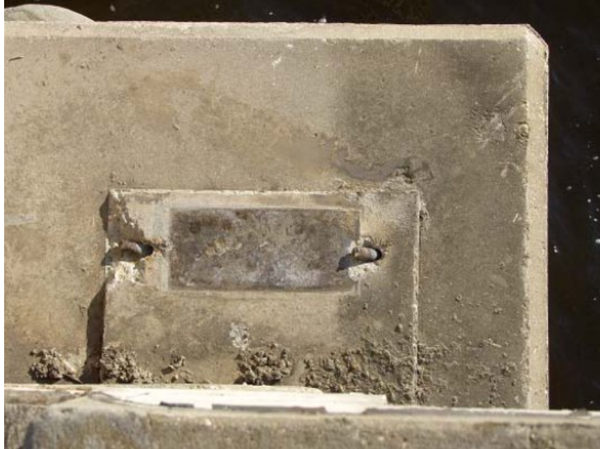
Figure 1- 7 I-10 Escambia Bay Bridge tie-downs damaged by Hurricane Ivan.
