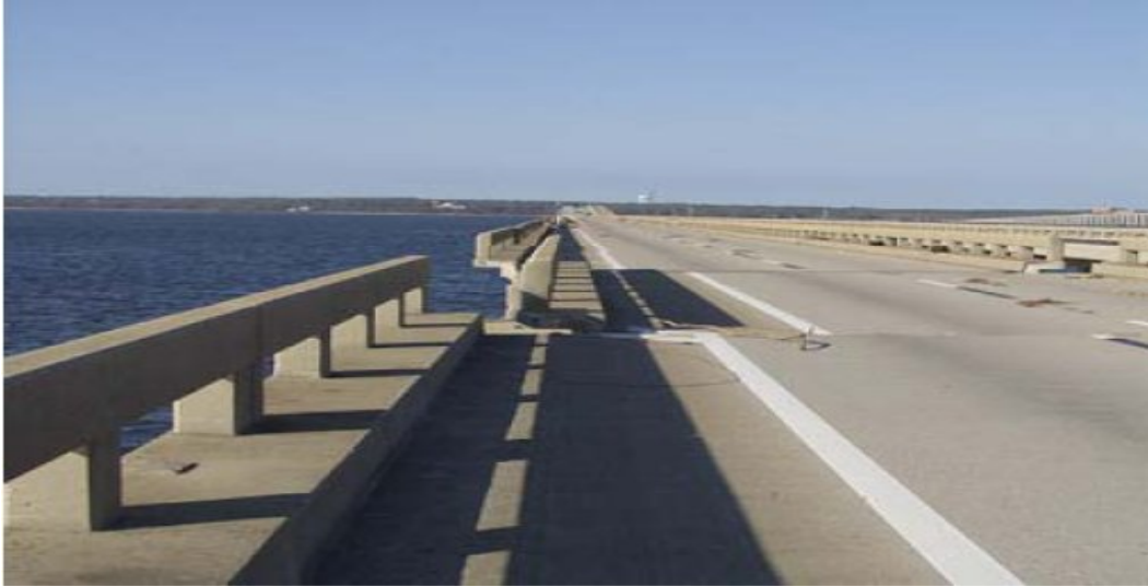
Figure 1- 5 I-10 - Escambia Bay Bridge spans displaced by Hurricane Ivan.
