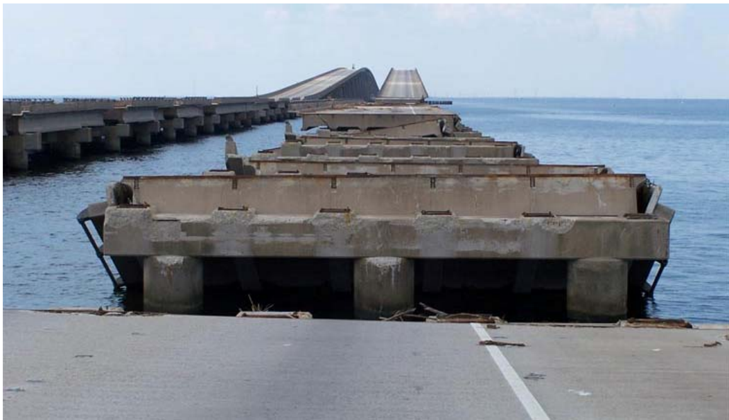
Figure 1- 10 I-10 Lake Pontchartrain Bridge spans removed by Hurricane Katrina.
