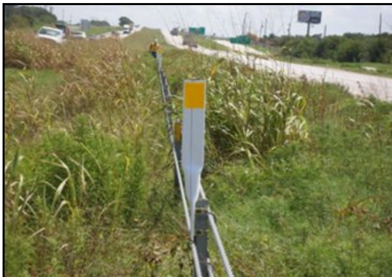
Figure 2-33. High Grass and Vegetation around a Cable Barrier System.
