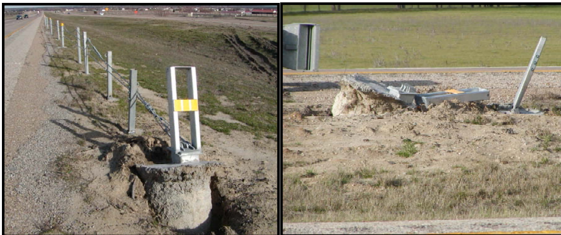
Figure 2-36. Example Photograph of Anchor Terminal Failure System in Texas.
