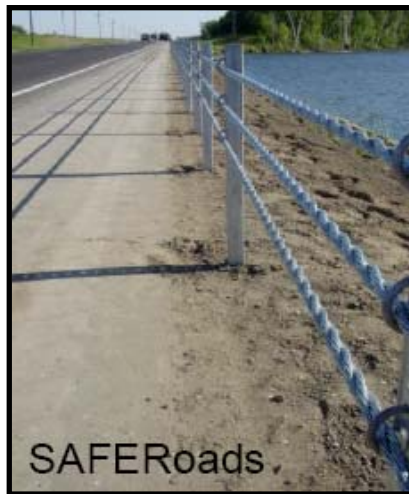
Figure 2-8. Nucor SAFERoads Cable Barrier System.
