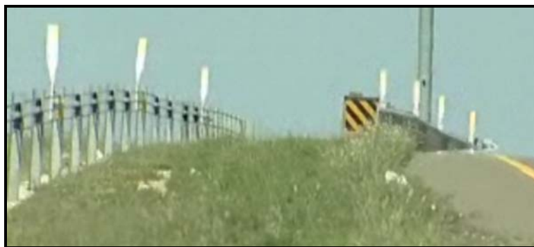
Figure 2-38. Picture Showing Special Extended Delineators.
