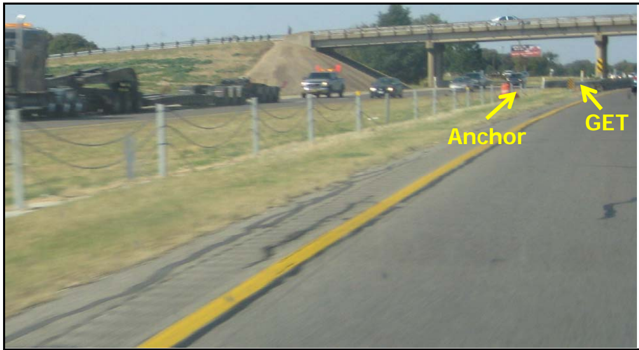
Figure 3-9. Example of Consequence of Having Anchor Terminal Unprotected.
