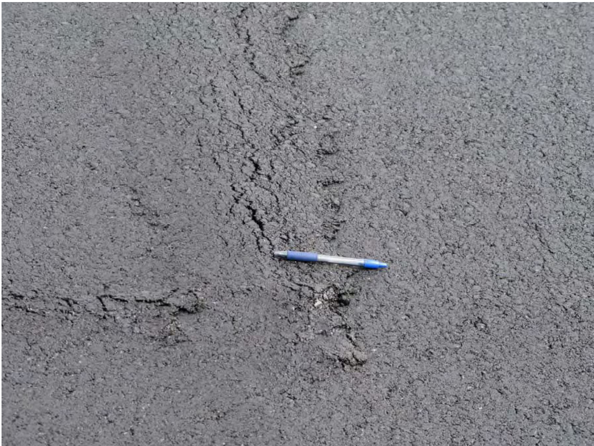
Figure 13. Bump and Transverse Cracks Over Crack 271
