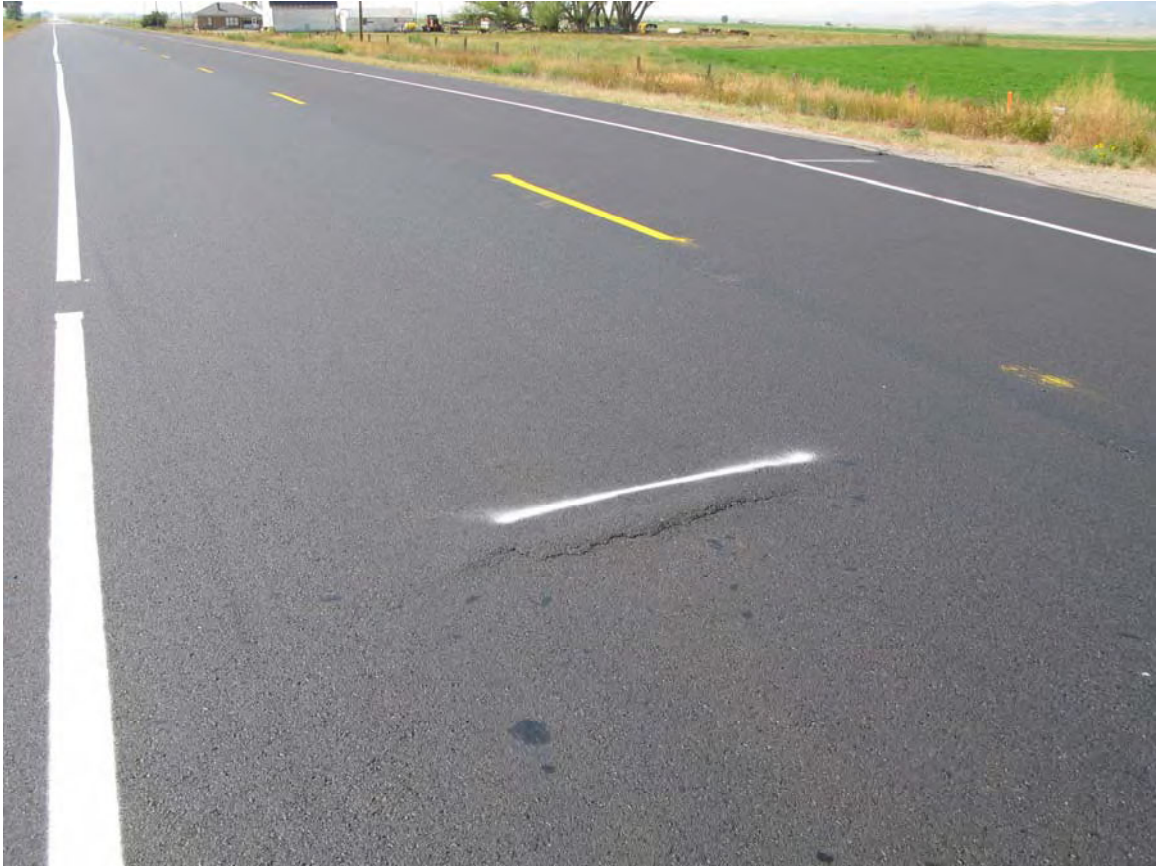
Figure 12. Bumps and Transverse Cracks at Station 150+00
