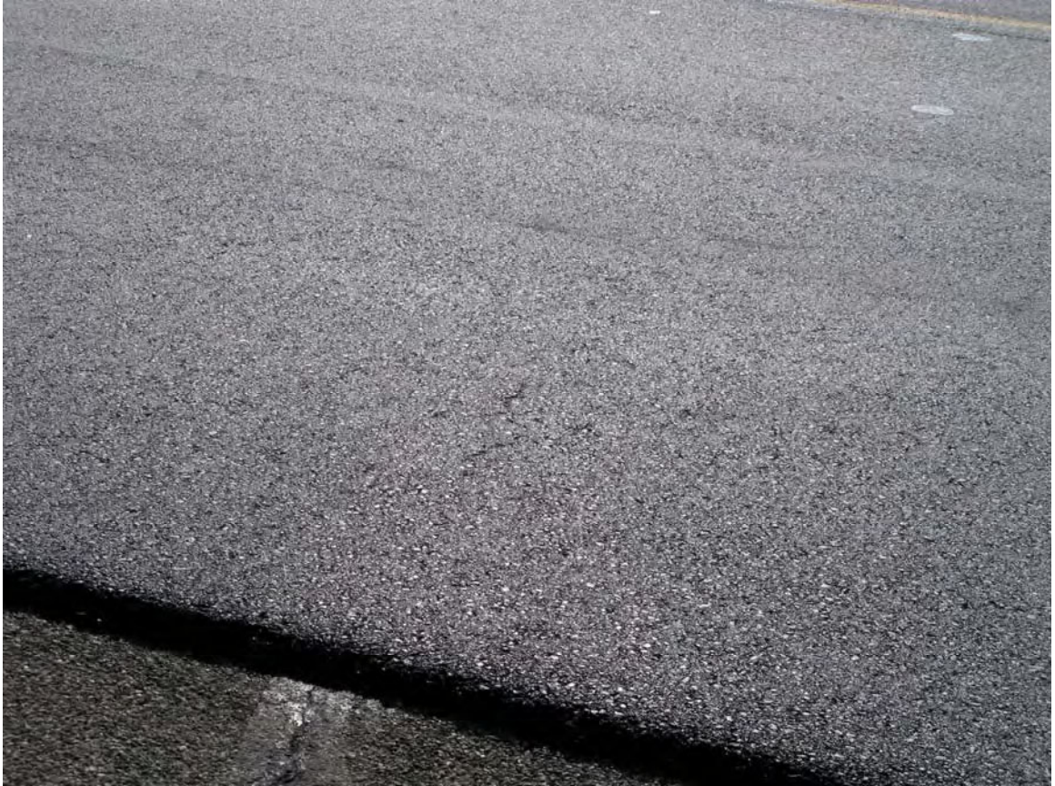
Figure 15. Transverse Crack Forming Over Crack 201 Northbound
