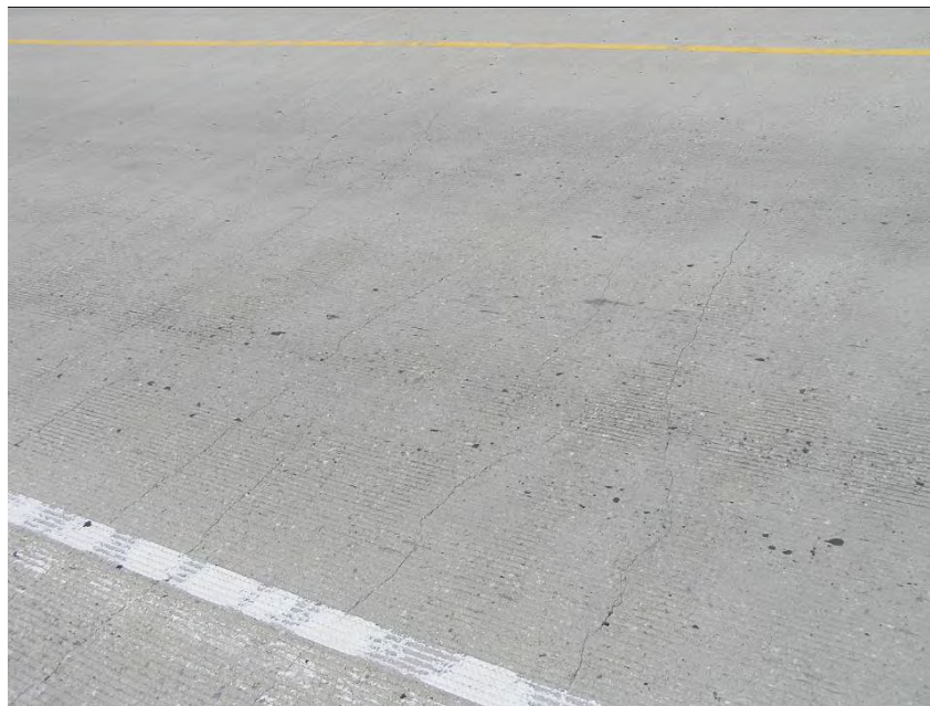
Figure 12. View of transverse cracking at structure F-15-BZ
