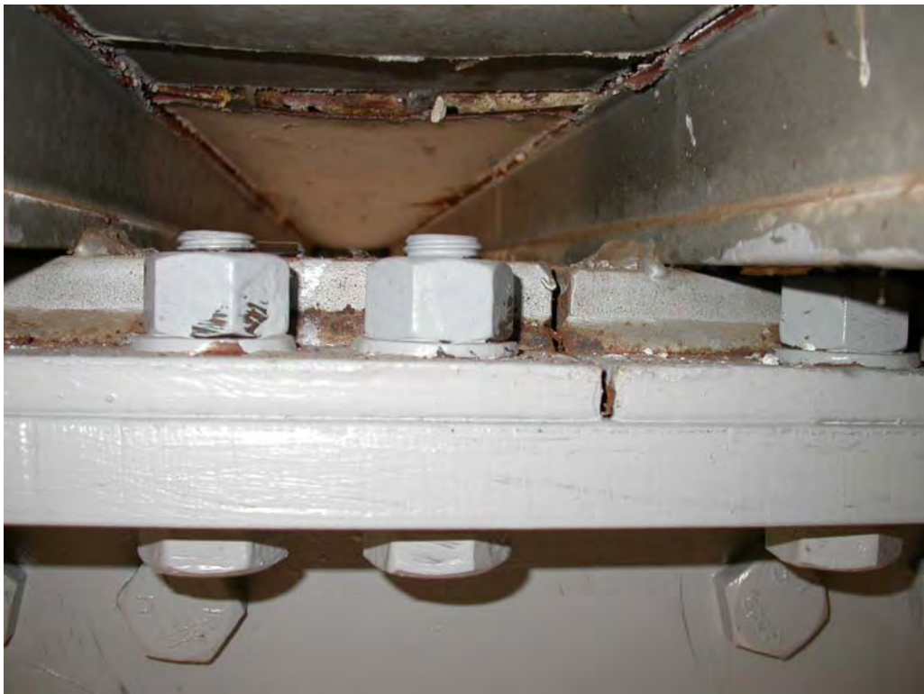
Figure 3-4. Close-up view of crack area after repair. *Note that fillet weld runs across shim plate butt joint.
