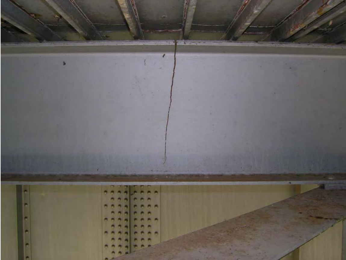
Figure 3-1. Cracked stringer found during 2005 inspection.
