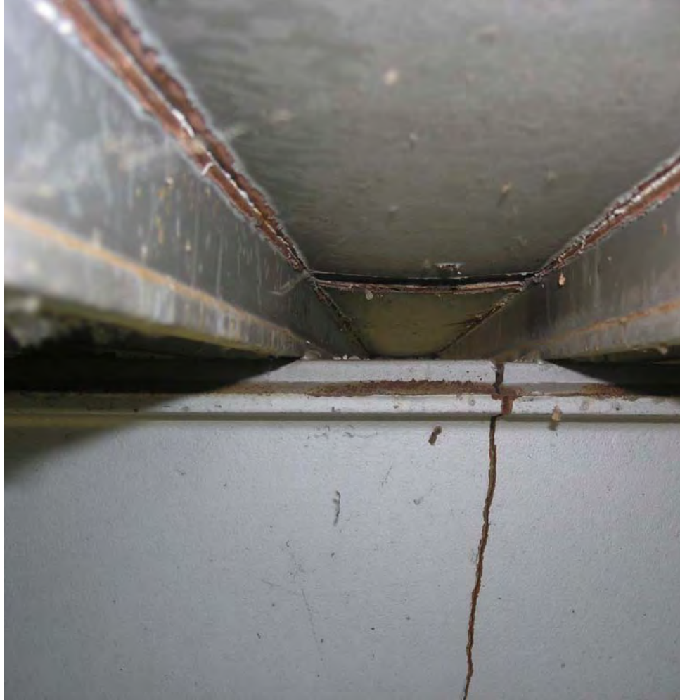
Figure 3-2. Close-up view of shim plate butt joint and crack.
