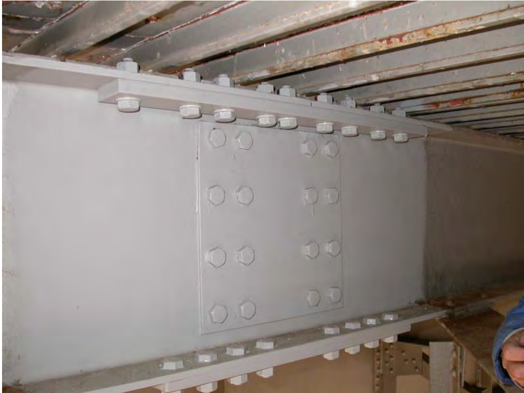
Figure 3-3. Splice repair of cracked stringer.
