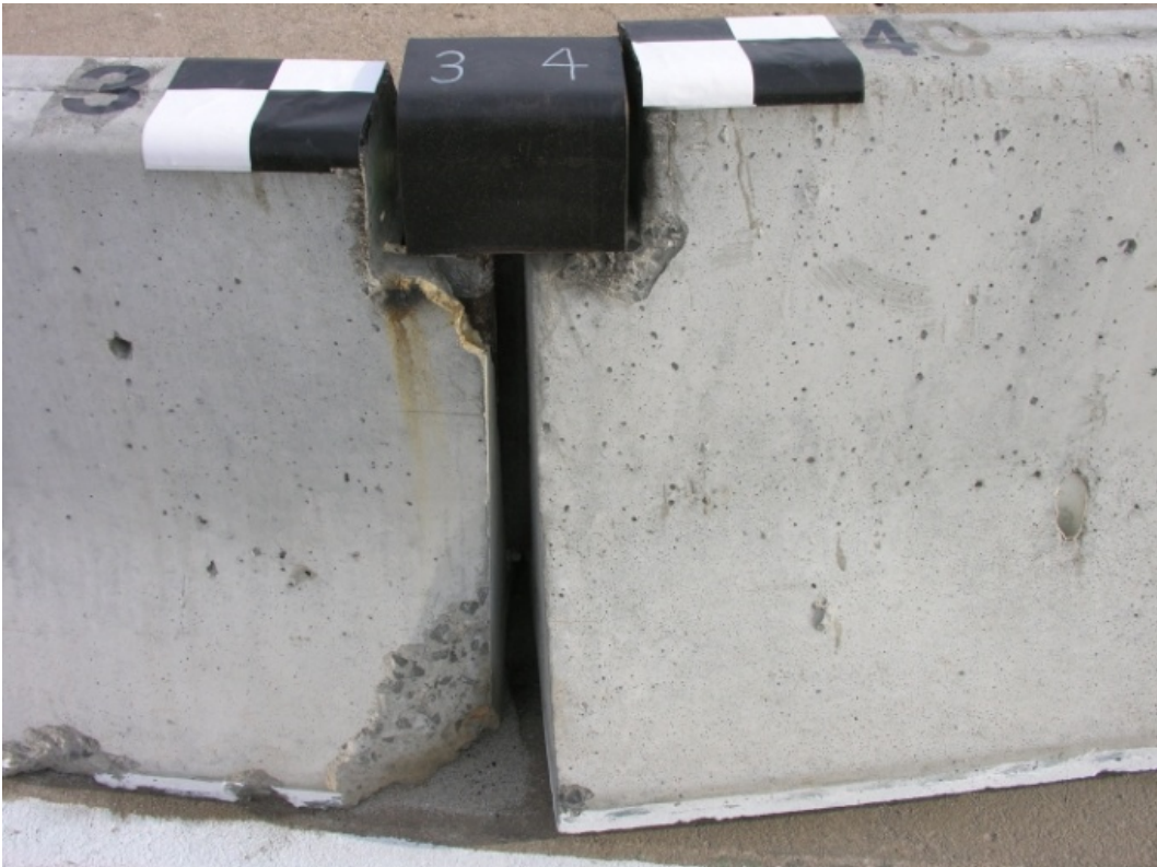
Figure 29. Joint 3-4 Connection Damage, Test NYTCB-4
