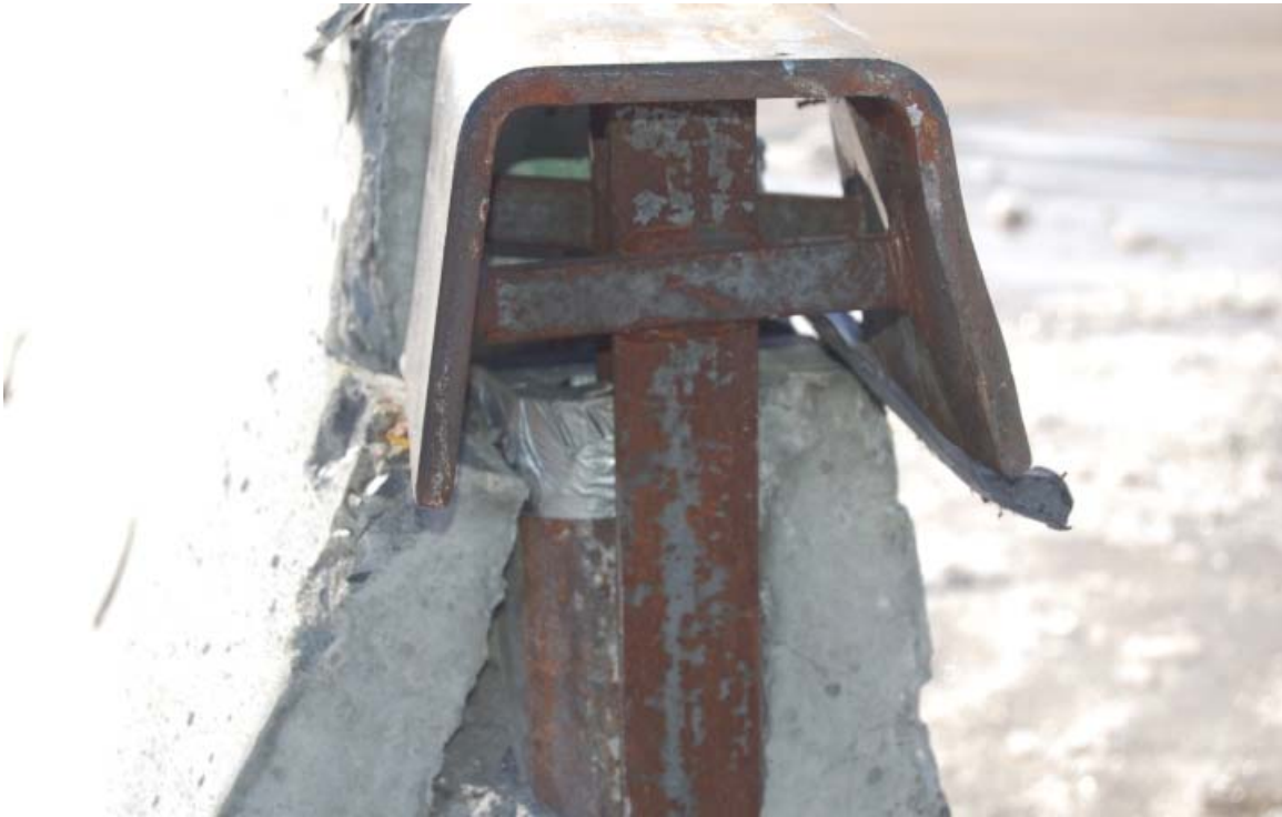
Figure 31. Joint 4-5 Connection Damage (Cont'd), Test NYTCB-4
