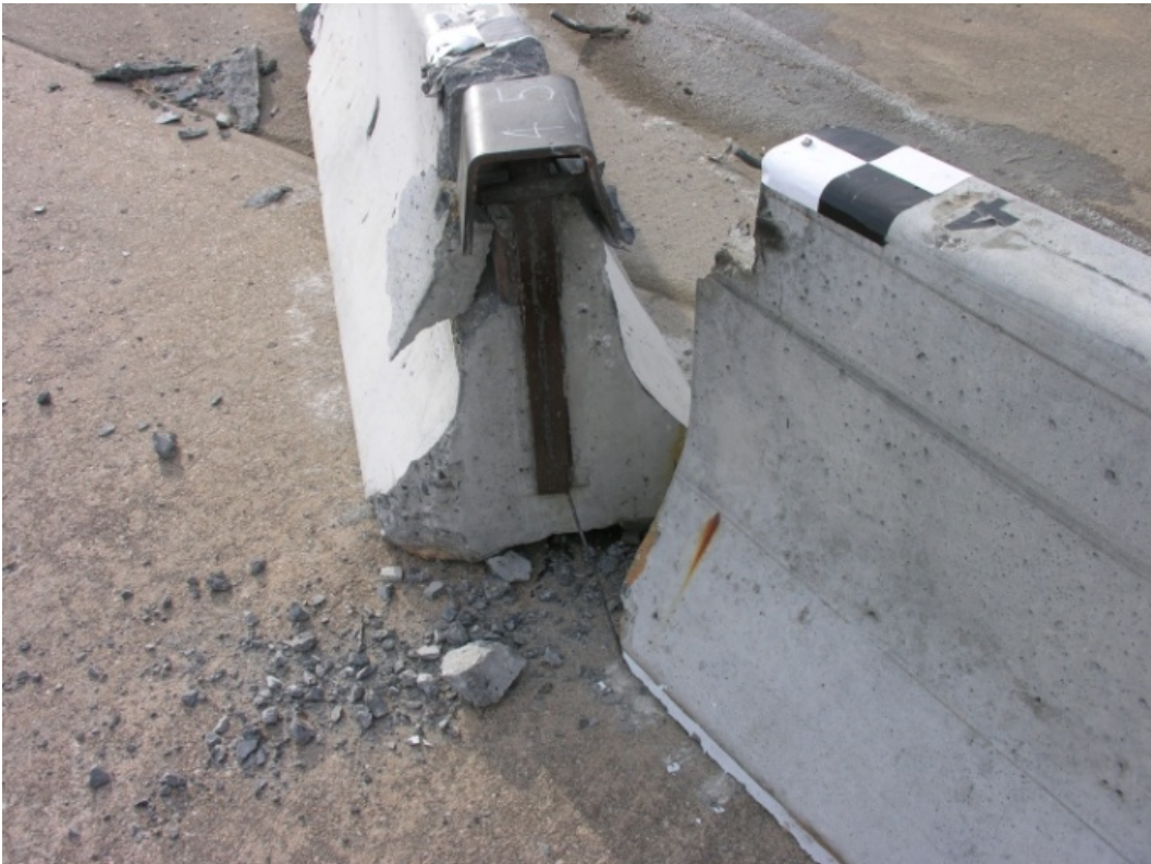
Figure 30. Joint 4-5 Connection Damage, Test NYTCB-4
