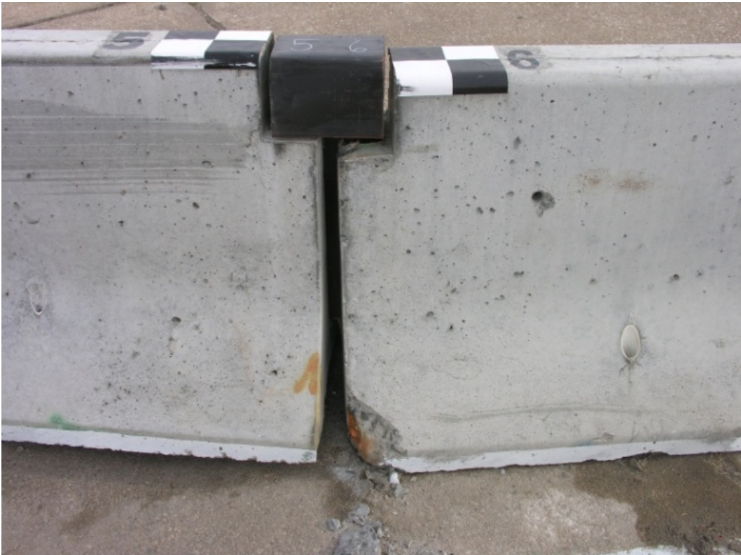
Figure 32. Joint 5-6 Connection Damage, Test NYTCB-4
