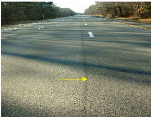
Photo 12: Crack in 4 inch Section – I87
