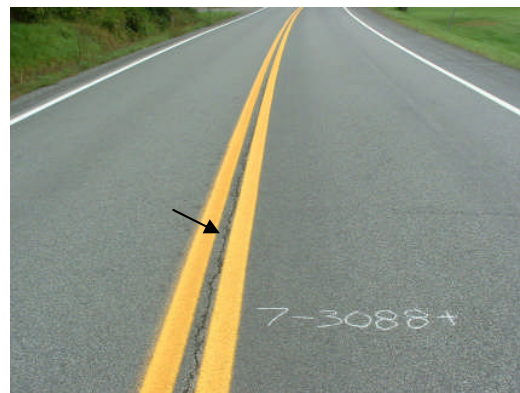
Photo 15: Cracking in Adhesive Section – Route 7
