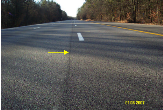
Photo 10: Crack in Control Section – I87
