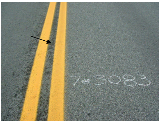
Photo 14: Ravelling Along Centerline – Route 7
