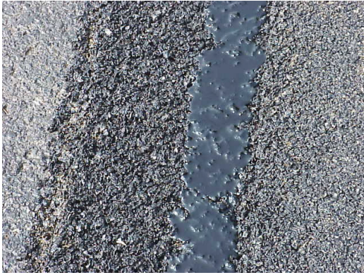
Photo 7: Adhesive on Top Edge of Wedge Jt.
