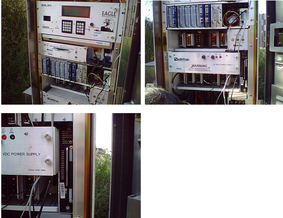
Figure 27 Pictures of the equipment cabinet at the Wade Road and Route 7 intersection
