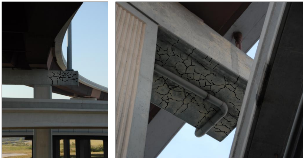
Figure 6-2: Signs of Deterioration within Connection Ramp Structures
