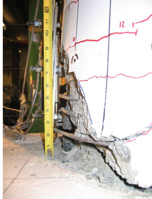
Figure 4-16. LB6-PT: Bar V00 fractured, Cycle 33 (6.75%).
