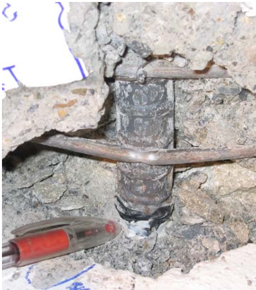
Figure 4-6. LB7-PT: Bar V18 buckling and spiral necking, Cycle 32 (5.43%).
