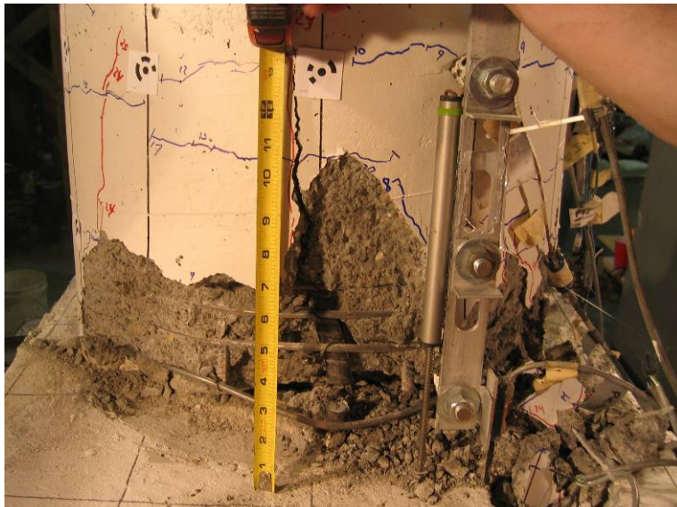
Figure 4-17. LB6-PT: Maximum spall height at end of test, Bar V18 fractured, Cycle 34 (-6.61%).
