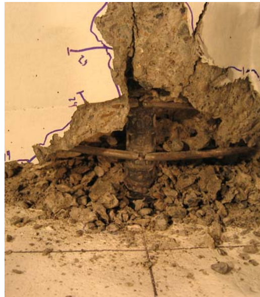
Figure 4-7. LB7-PT: spiral fracture, Cycle 32 (-5.32%).
