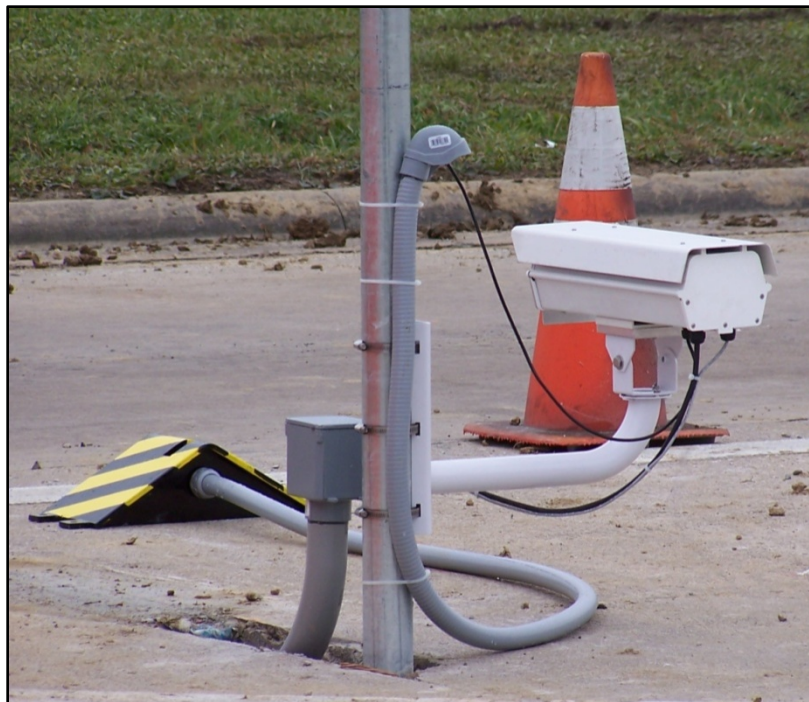
Figure 2. Photo. Passenger side components of the SIRIS system.
