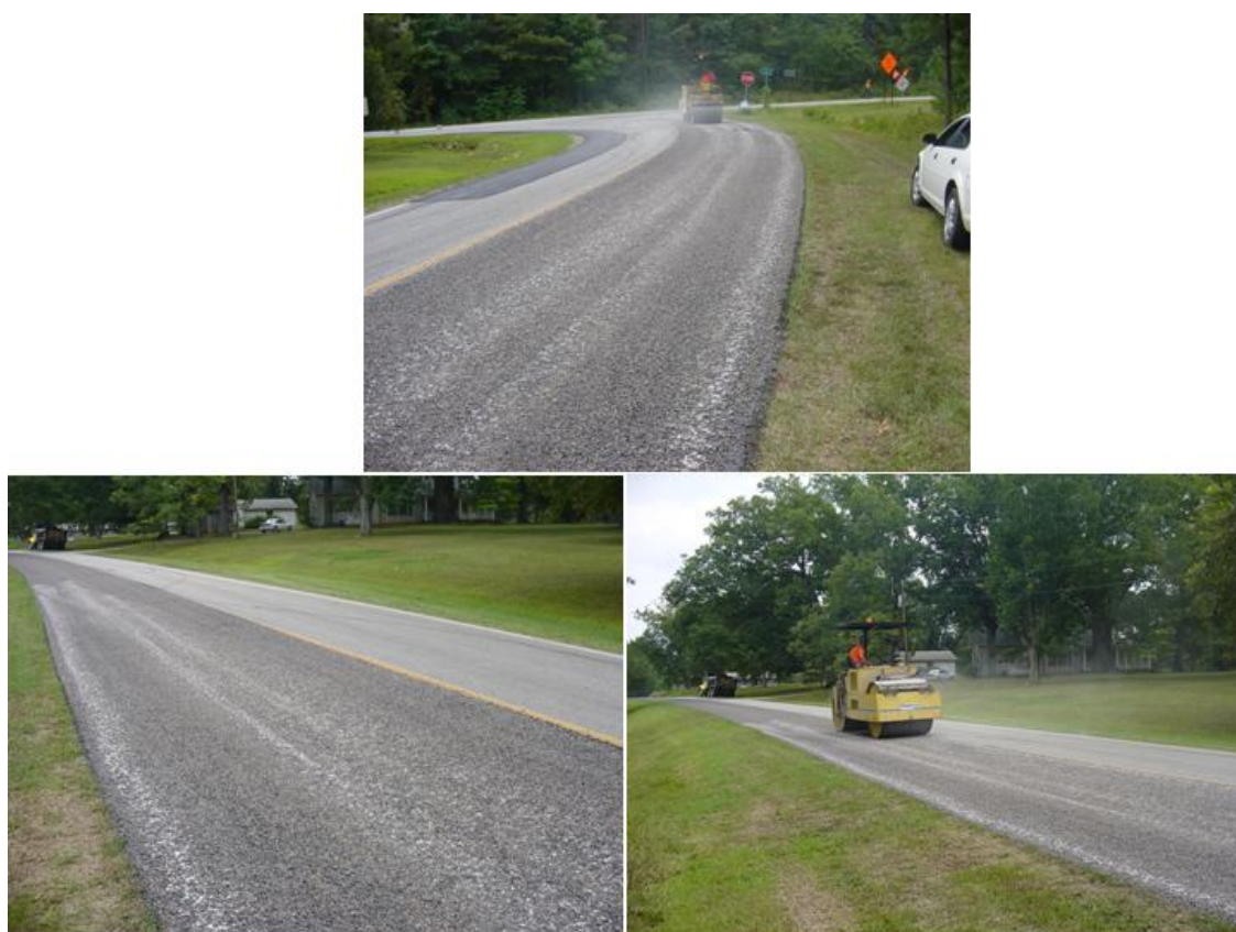
Figure 4-6 Uneven compaction under steel wheel roller
