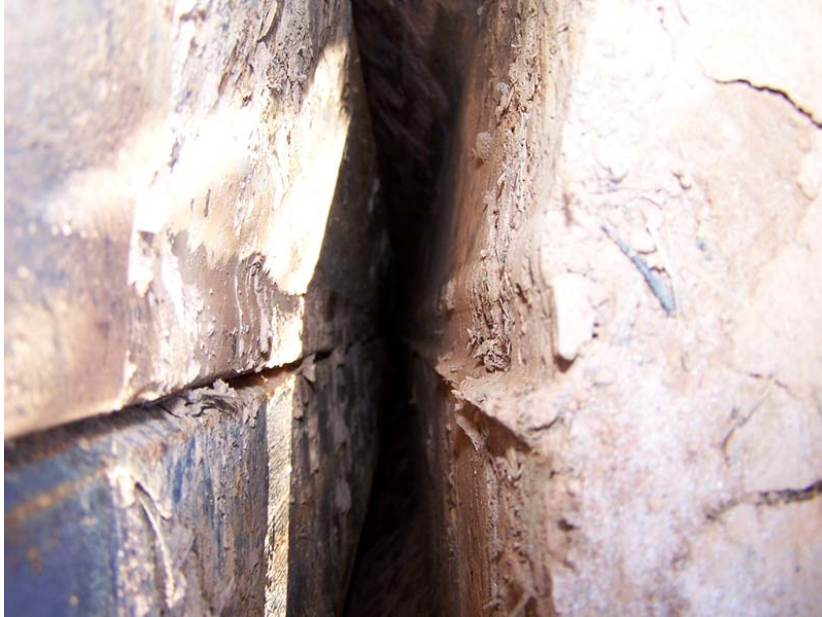
Figure 6.3 - Disconnection of sheet piles from soil mass
