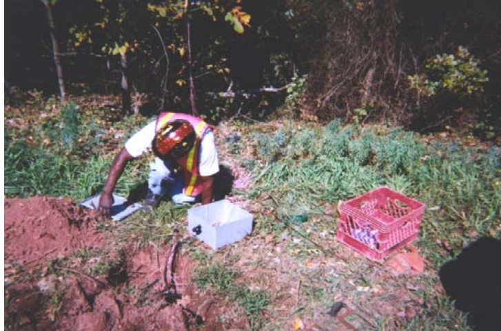
Figure 64 Photograph of control/junction box linked to sensor wires and ready to be buried.
