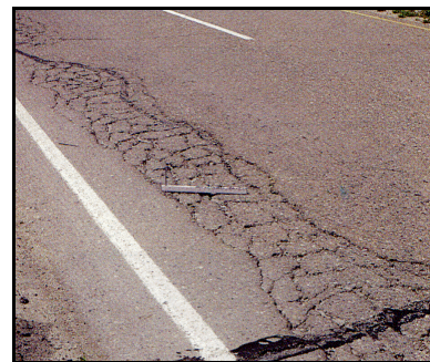
HMA with Alligator Cracking
