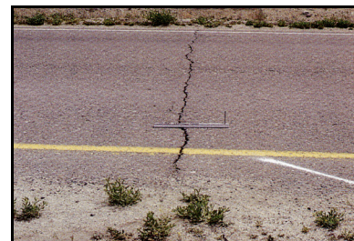
HMA with transverse cracking
