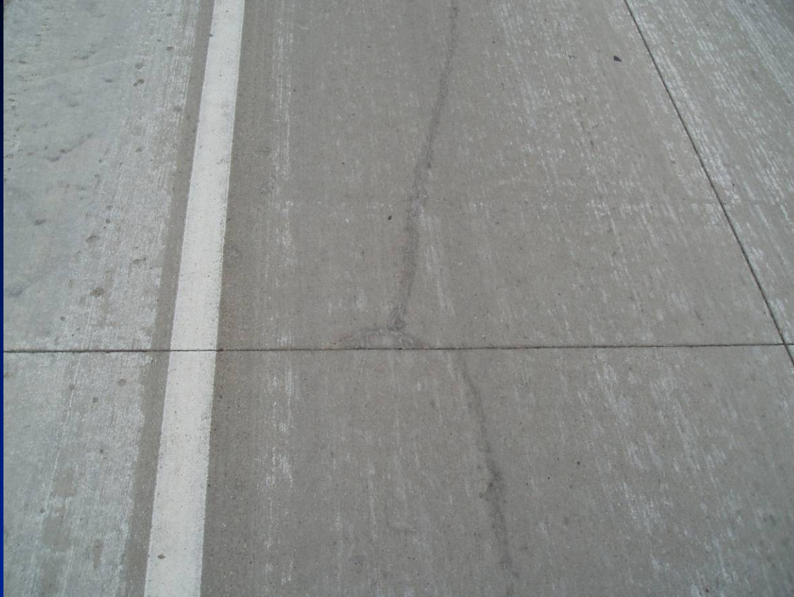
Iowa 175 Longitudinal Crack (widening related)
