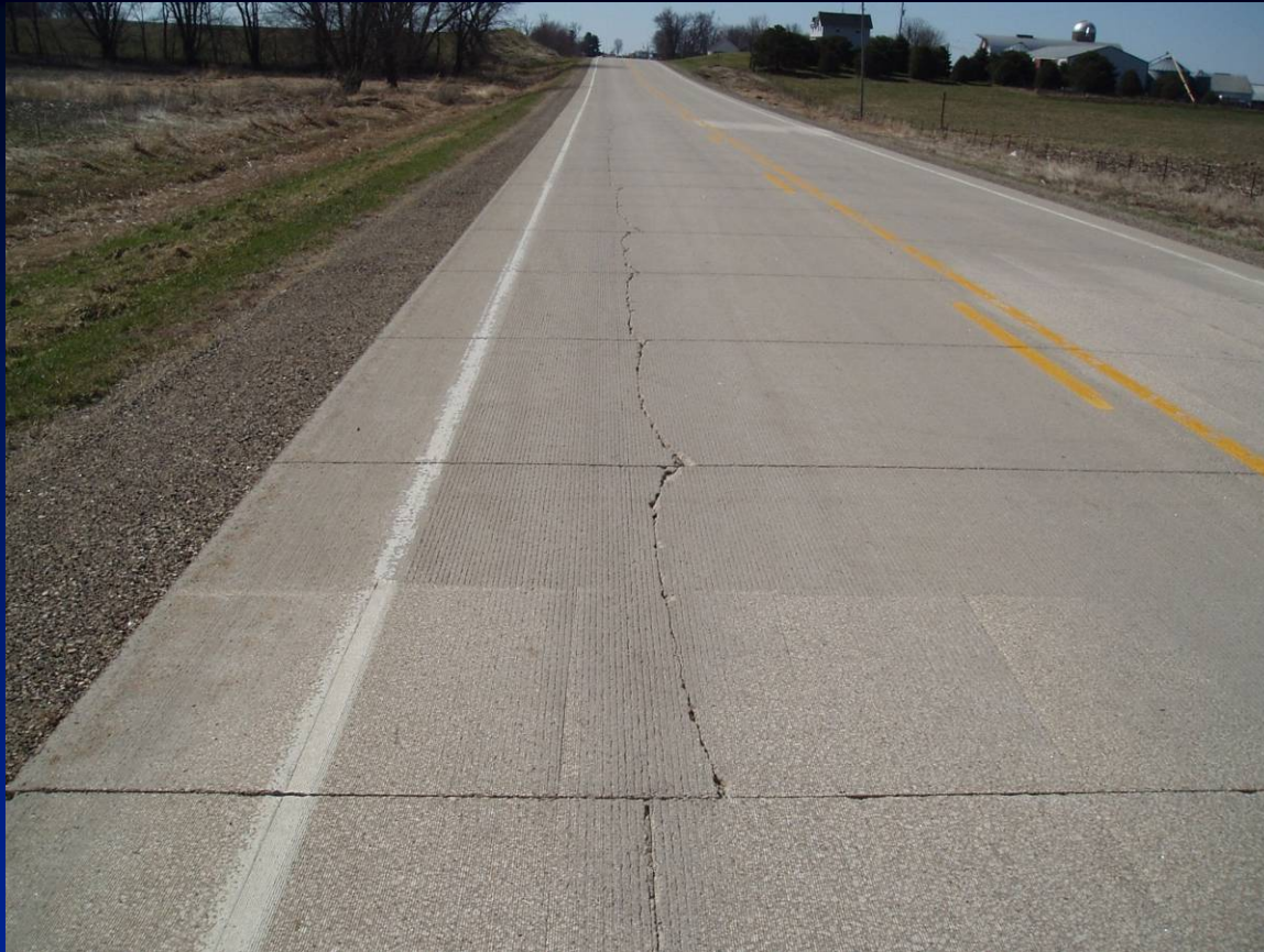
Iowa 13, longitudinal Crack (Knife and widening related)
