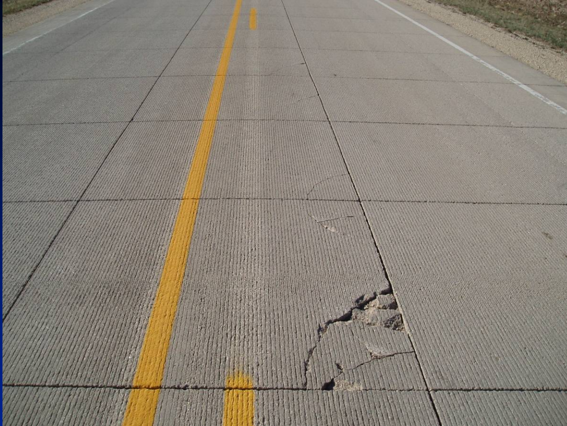
Iowa 13, Interior Corner Crack
