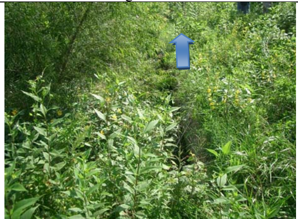
The culvert exit was covered by vegetation
