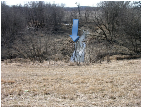
The stream is fairly well aligned with the culvert. Steep slopes from all the culvert sides cut strong ditches merging upstream the culvert.
