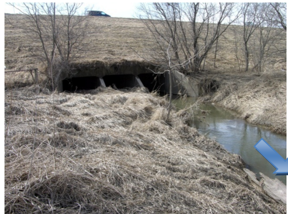
Constant sedimentation level though the more than 50m culvert length is blocking the two culvert boxes.
