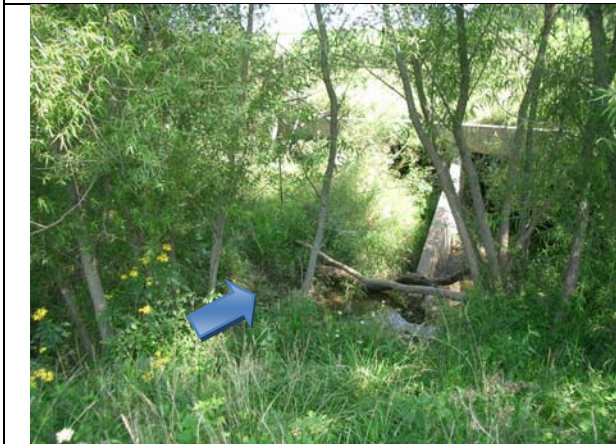
Three-barrel culvert with two barrels blocked by debris and sediment.
