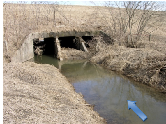
Considerable clogging appears on the right and central boxes of the culvert. The left box is clean; the others are heavily sedimented (about 1 m elevation difference).
