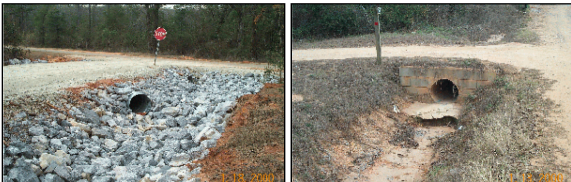
Figure 2-1-2 Cross drains usually connect road ditches on the side of a roadway
