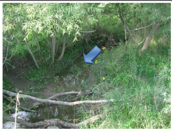
View from culvert center. The approach channel is not well aligned with the culvert
