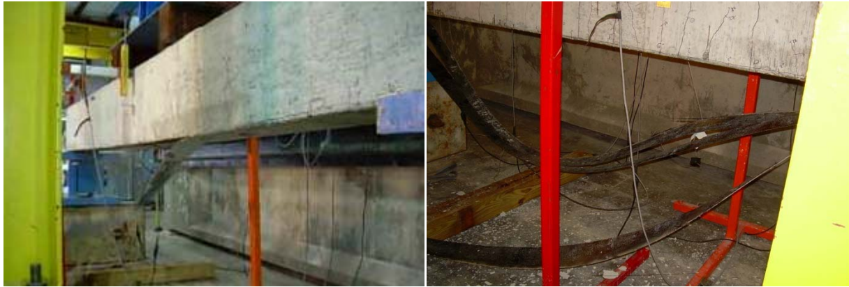
(a) Initial Failure via Debonding
