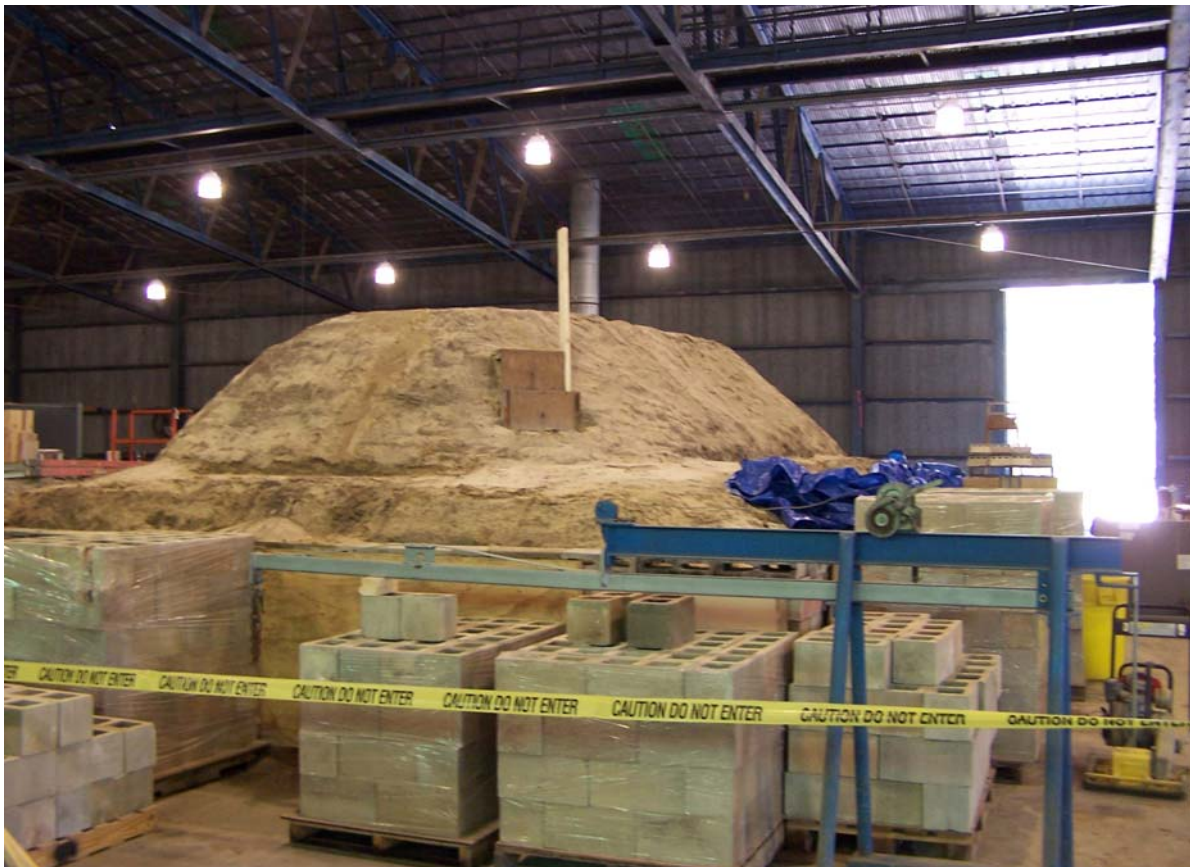
Figure 18. End restraining blocks.
