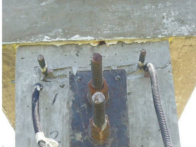
Figure 126 – Cracks around PT anchorage.
