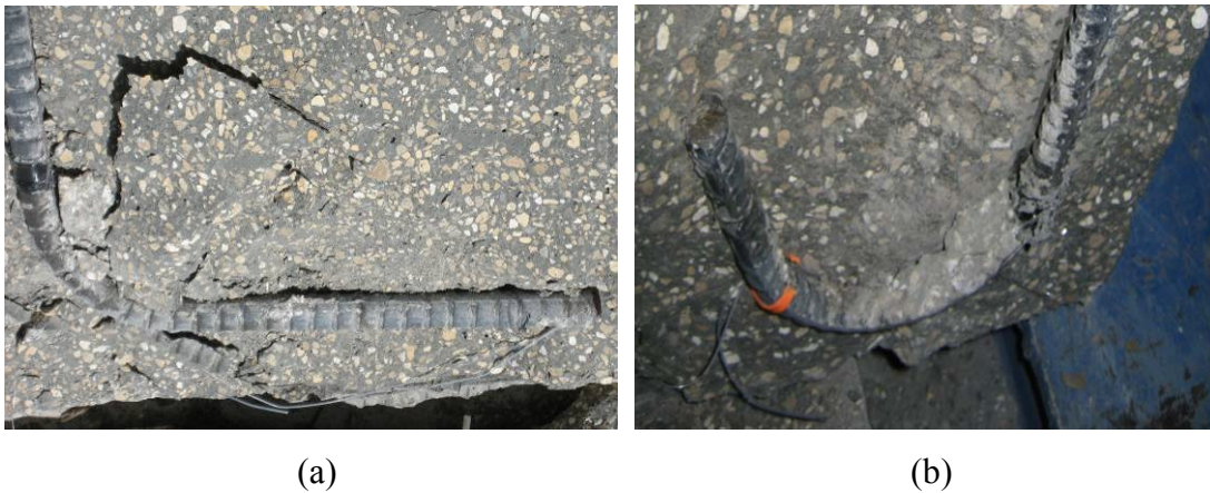
Figure 28. Crushed concrete inside of bend radius (a) 90 deg. hook and (b) 180 deg. hook.
