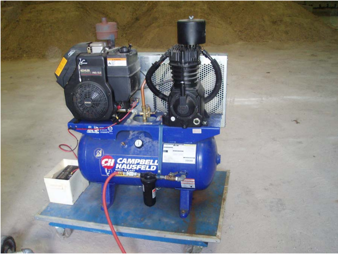
Figure D-10. Photo Showing 175 psi Air Compressor.
