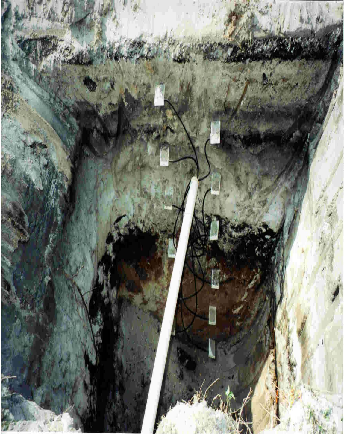
Figure B.3 Cross Sectional View of the TDR Installation in Field Test Pit
