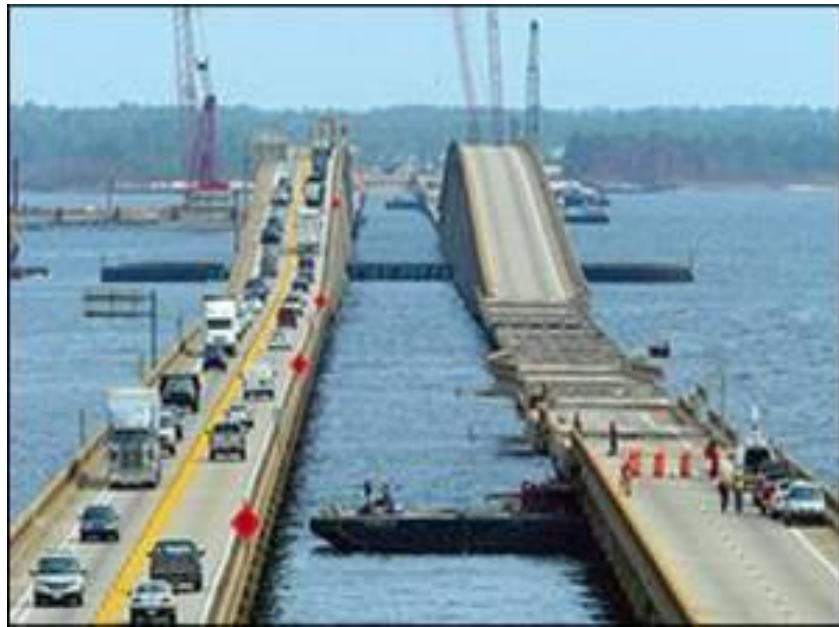
Figure A-25. Westbound bridge opens to traffic (Courtesy of FDOT and William Nickas)
