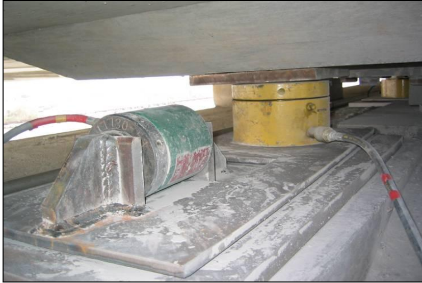
Figure A-17. 200-ton jack used to lift and align the main span (Courtesy of Brasfield & Gorrie)
