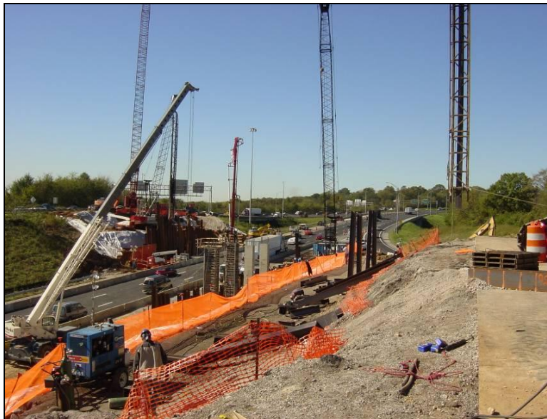
Figure A-8. First week: clean up and placement of steel piling (Courtesy Brasfield & Gorrie)
