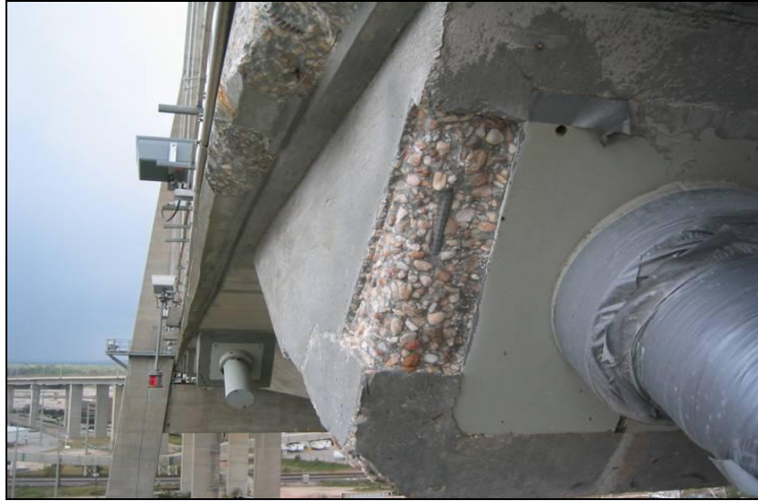
Figure A-15. Damage to the superstructure concrete (Courtesy of Brasfield & Gorrie)
