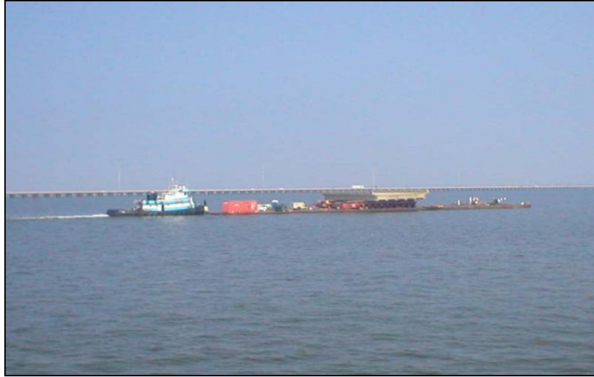
Figure A-36. Spans switch from westbound to eastbound bridge (Courtesy of LADOTD and Paul Fossier)
