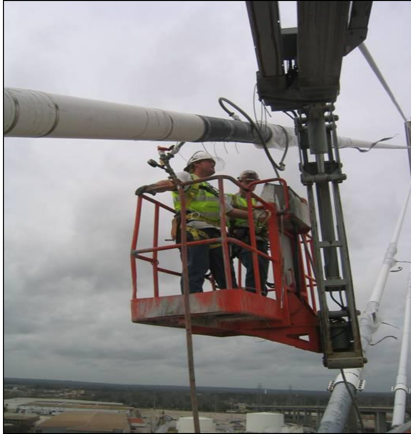
Figure A-16. Lift truck with basket used to repair cable stays (Courtesy of Brasfield & Gorrie)
