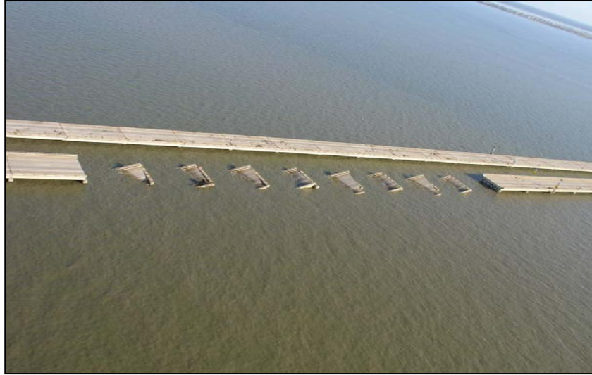
Figure A-29. Bridge damages (Courtesy of LADOTD and Paul Fossier)
