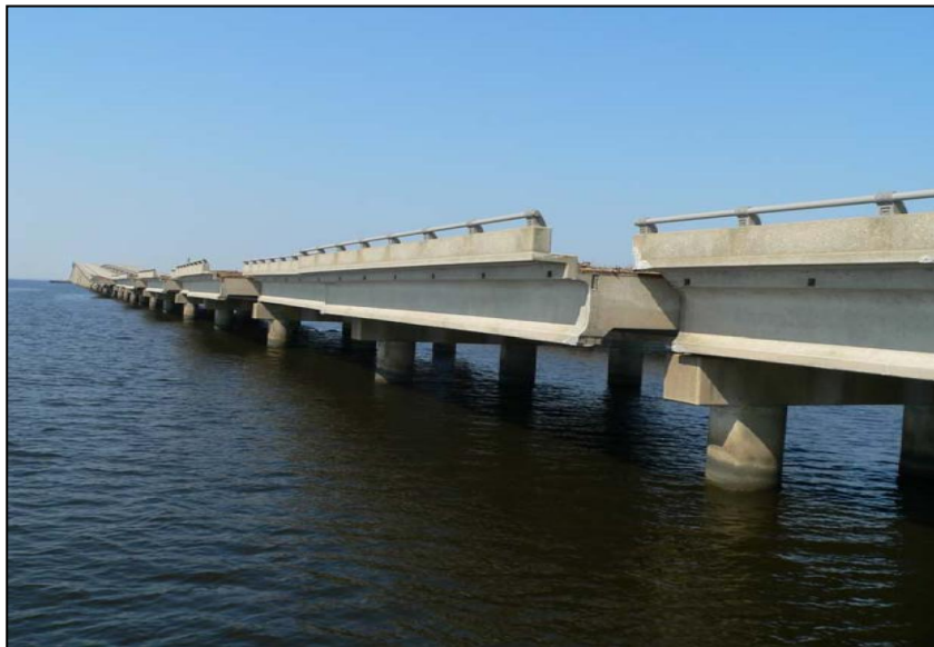
Figure A-31. Span displacement (Courtesy of LADOTD and Paul Fossier)
