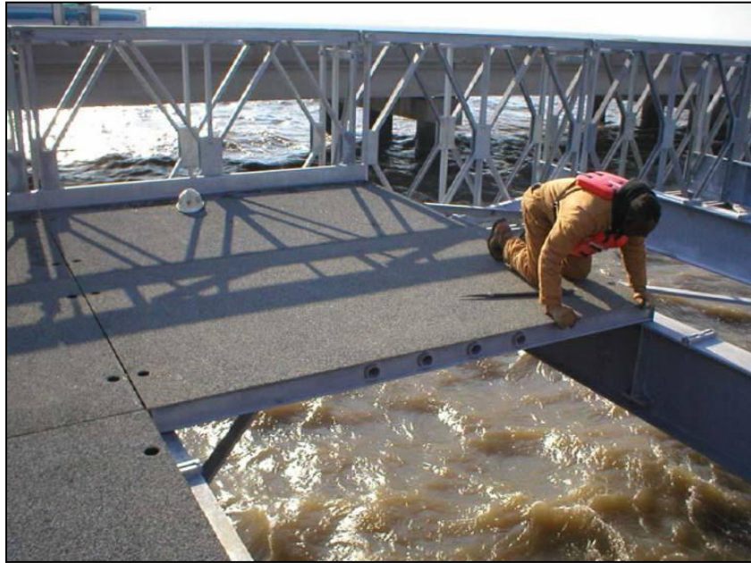
Figure A-38. Acrow 700 series steel panels (Courtesy of LADOTD and Paul Fossier)
