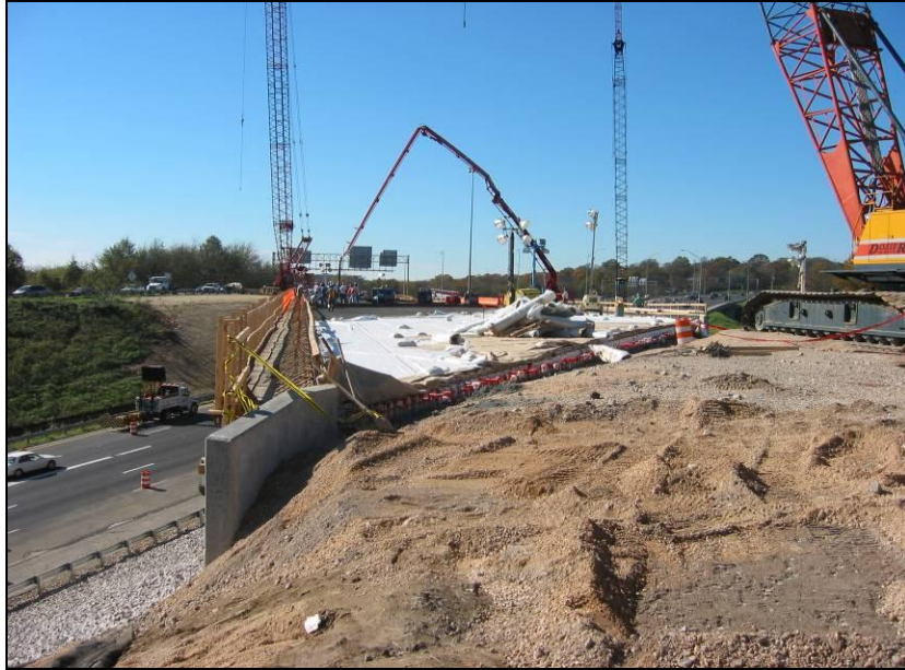
Figure A-11. Fourth week: reinforced concrete bridge deck (Courtesy of Brasfield & Gorrie)
