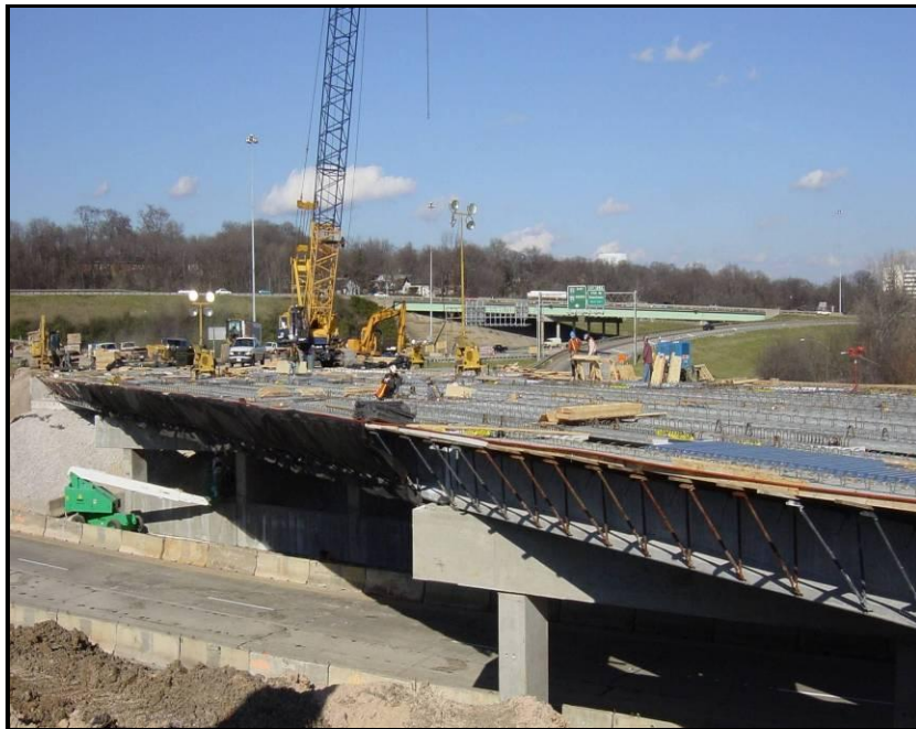
Figure A-4. Third week of construction: concrete girders and reinforced concrete deck (Courtesy of Brasfield & Gorrie)
