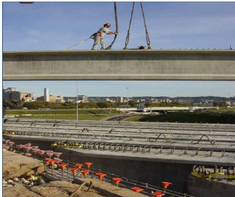
Figure A-10. Third week: girders were placed on the bridge (Courtesy Brasfield & Gorrie)
