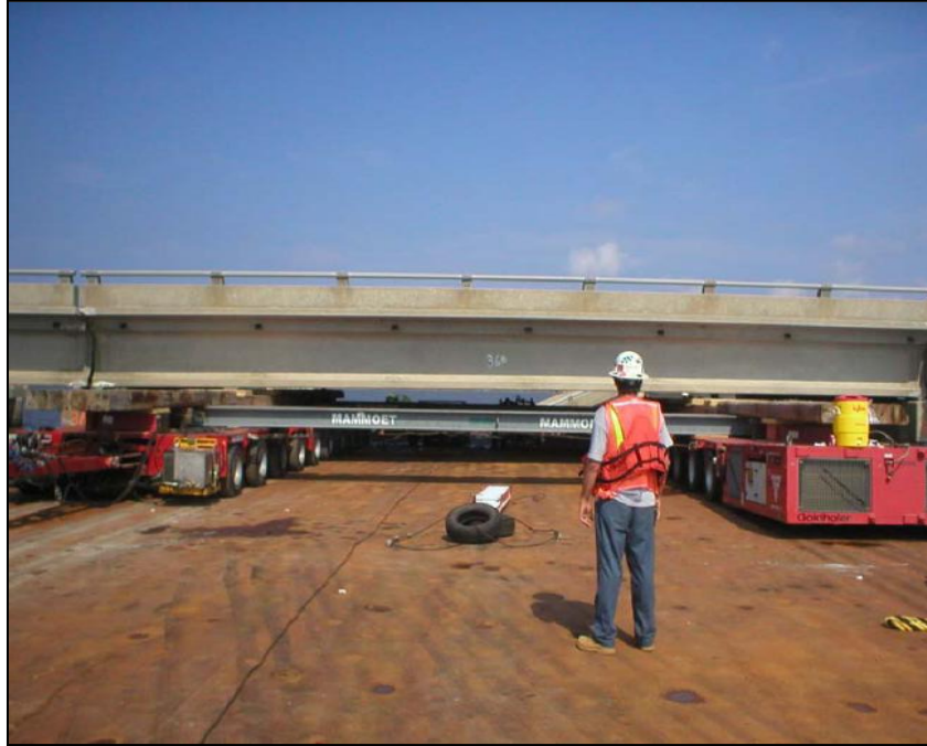
Figure A-34. Realignment of spans using SPMT (Courtesy of LADOTD and Paul Fossier)
