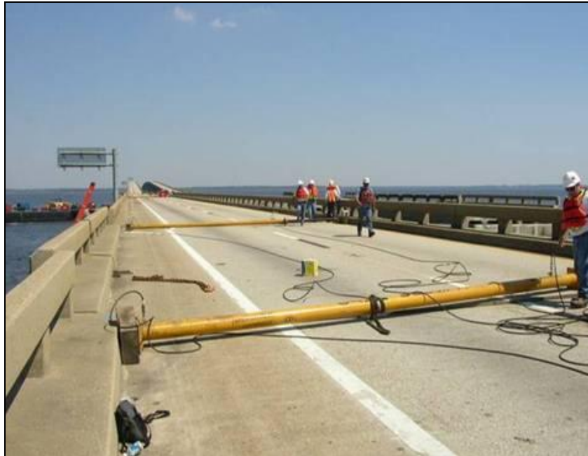
Figure A-23. Span realignment by jacks and slide method (Courtesy of FDOT and William Nickas)
