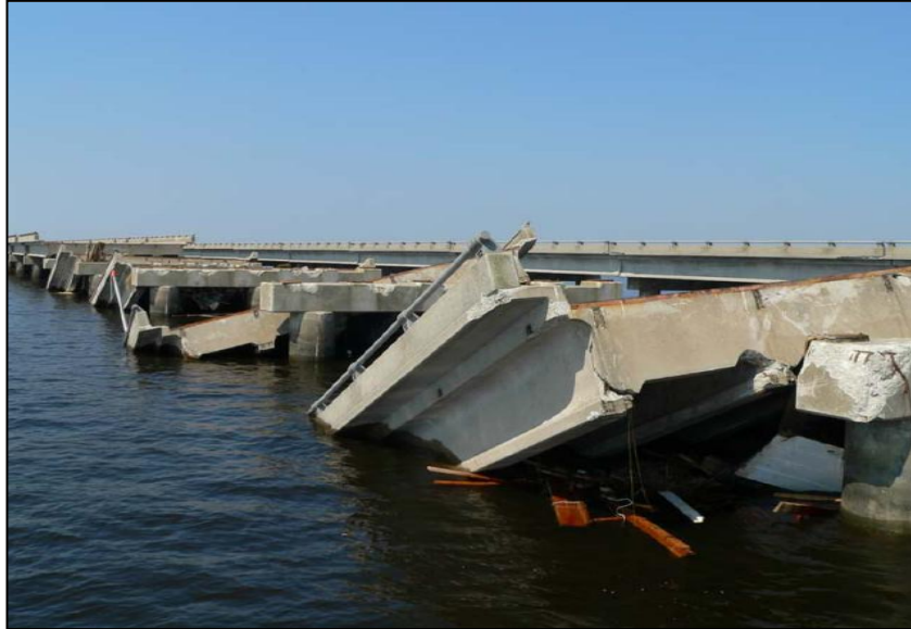
Figure A-30. Dislodged spans (Courtesy of LADOTD and Paul Fossier)
