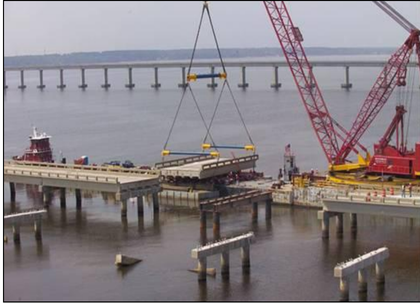
Figure A-24. Replacement spans using crane and SPMT (Courtesy of FDOT and William Nickas)
