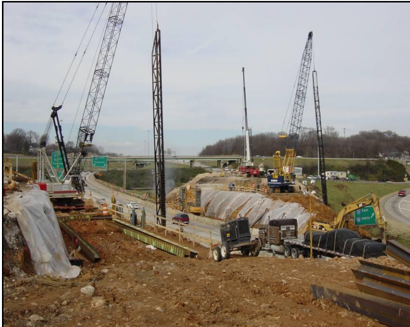
Figure A-2. First week of construction: materials and equipment (Courtesy of Brasfield & Gorrie)
