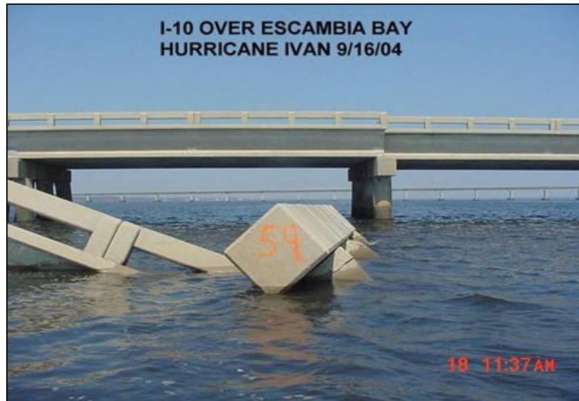
Figure A-22. Missing or destroyed pile bents (Courtesy of FDOT, William Nickas, and Thomas A. Andres)
