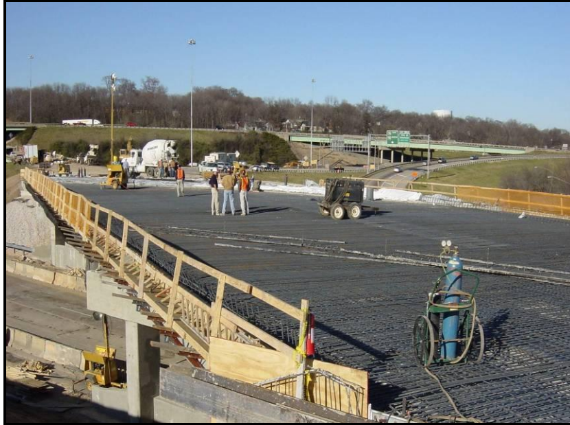
Figure A-5. Fourth week of construction: concrete deck reinforcement (Courtesy of Brasfield & Gorrie)
