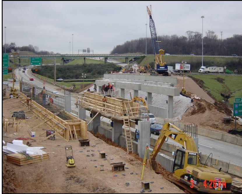
Figure A-3. Second week of construction: concrete caps and columns (Courtesy of Brasfield & Gorrie)
