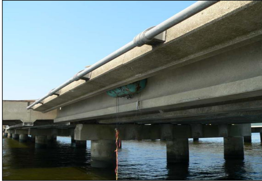
Figure A-32. Barrier damage (Courtesy of LADOTD and Paul Fossier)
