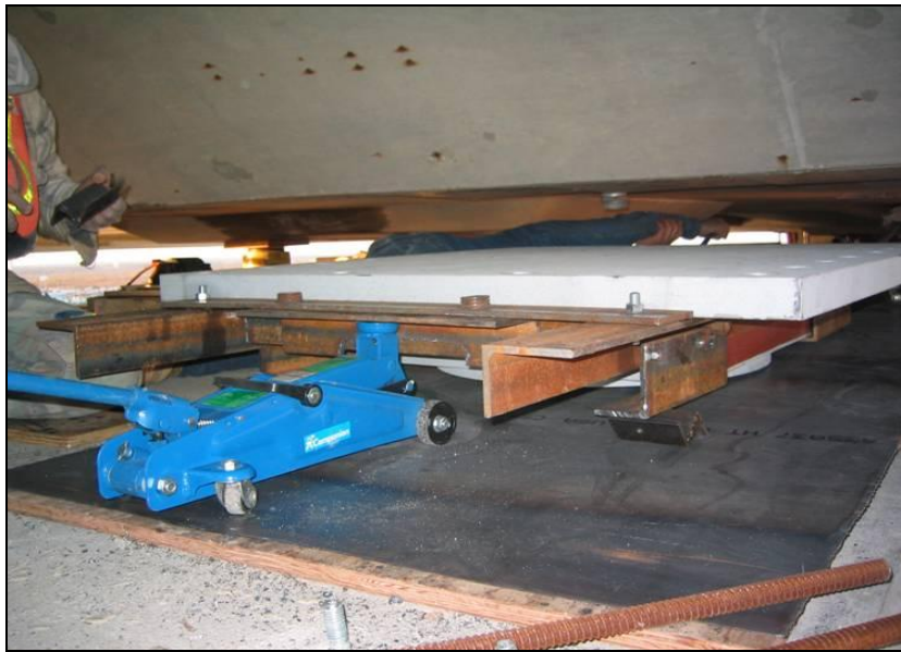
Figure A-18. Jacks used to lift and align the main span (Courtesy of Brasfield & Gorrie)
