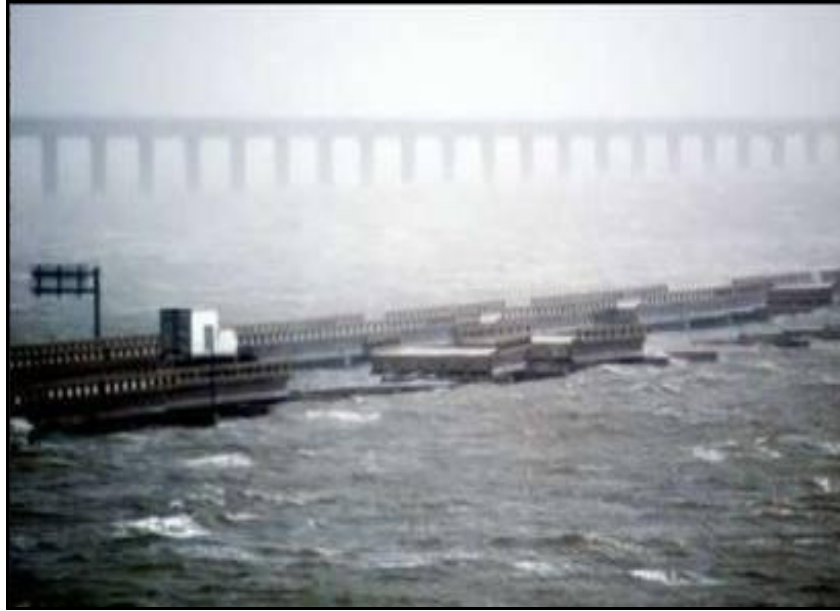
Figure A-19. Bridge damages (Courtesy of FDOT, William Nickas and Thomas Andres)
