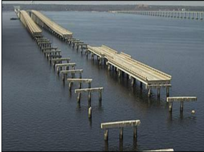
Figure A-20. The missing eastbound and westbound spans (Courtesy of FDOT, William Nickas, and Thomas A. Andres)
