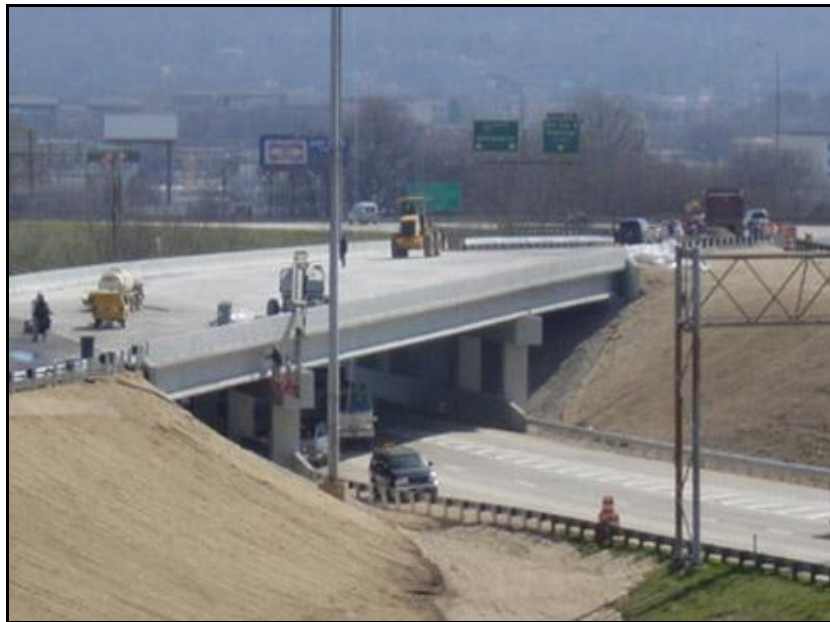
Figure A-6. Fifth week of construction: I-65 bridge complete (Courtesy of Brasfield & Gorrie)
