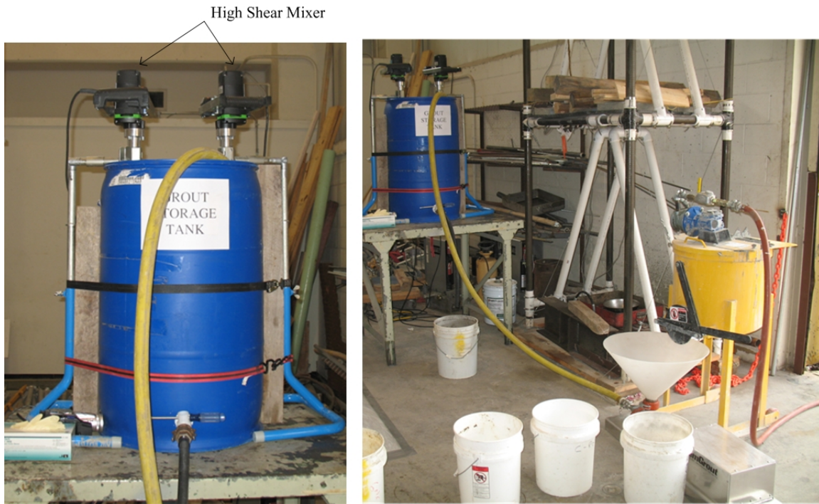
Figure B-4. Grout Storage Tank and High Shear Mixer.
