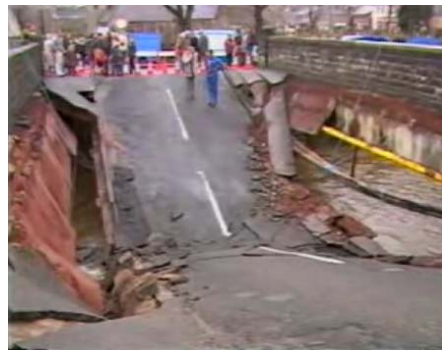
Figure 2-1. Collapsed Ynys-y-Gwas Bridge (YouTube 2009).
