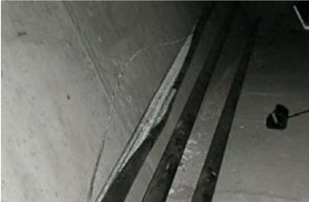
Figure A. Broken strands and broken ducts.
