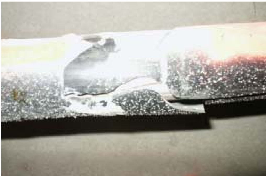
Figure F. Broken ducts and exposed strands.
