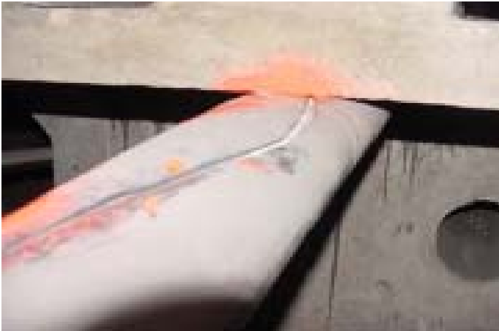
Figure D. Cracked ducts.
