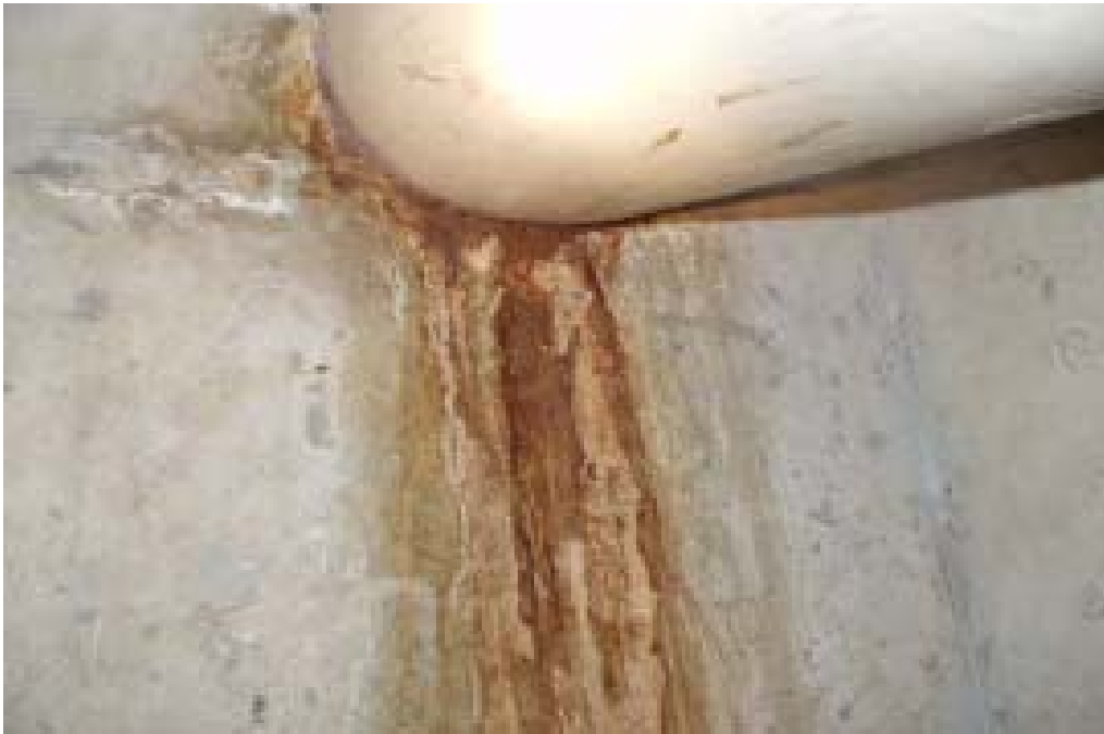
Figure O. Sign of past moisture infiltration in the concrete girder, broken drainage pipe.
