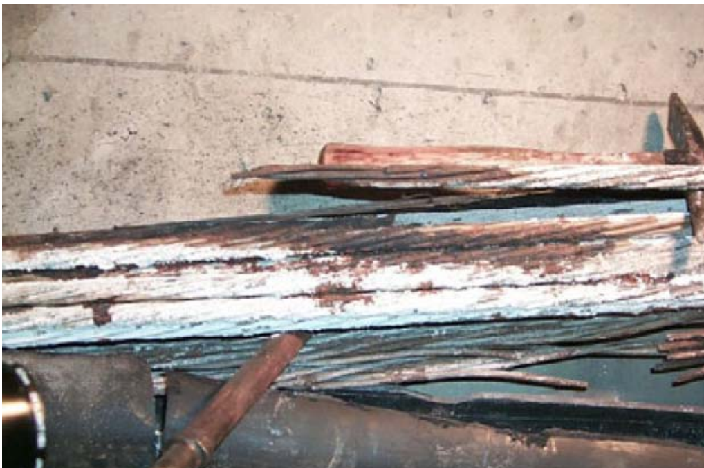
Figure B. Corroded and broken strands and broken ducts.
