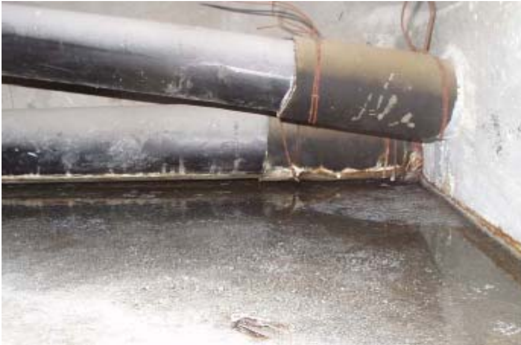
Figure M. Standing water in the concrete box girder.
