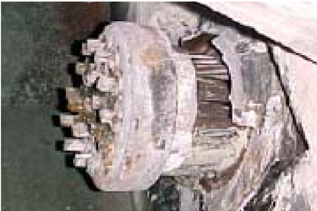
Figure J. Loose anchorage (indicating broken strands).
