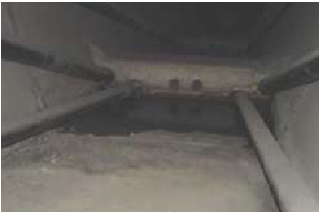
Figure N. Standing water in the concrete box girder.
