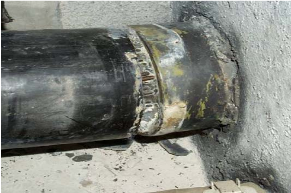
Figure E. Broken ducts and exposed strands.
