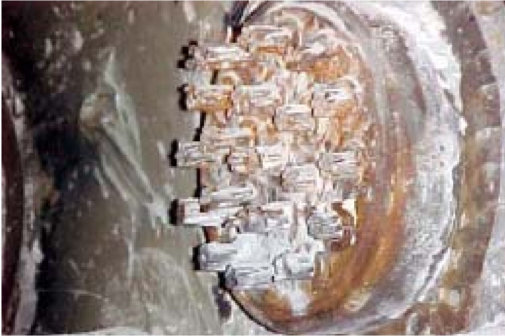
Figure I. Missing anchorage cap, exposed anchor head, and corroded strands.
