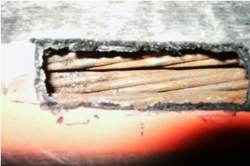
Figure H. Voids in tendons and corroded strands.
